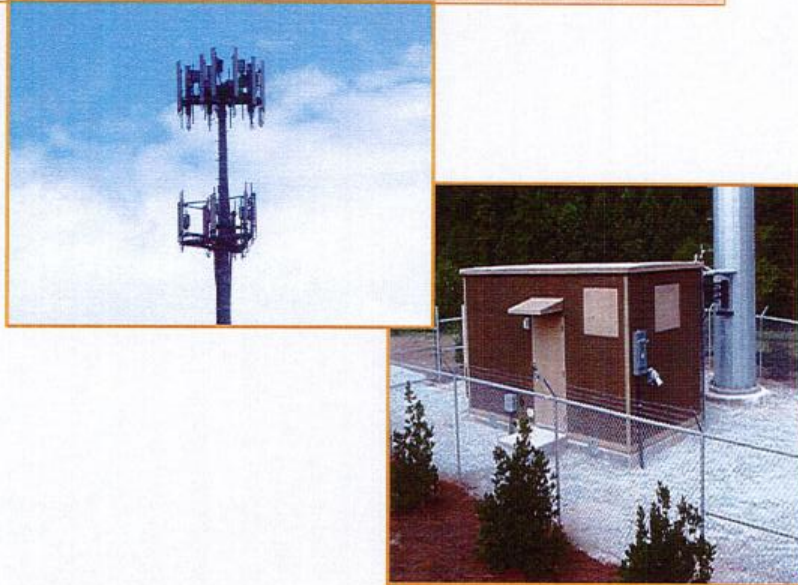
Typical Macro facility – industry standard sized colocateable facility with full compliment of radios
