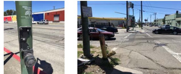
Exhibit I-1B: Northbound Approach With No Sidewalk; and Pedestrian Activation Button With No Signage
