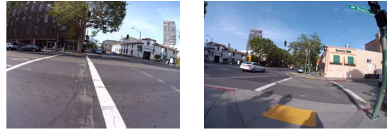
Exhibit I-4B: Degraded Pavement; Permissive Left Turn on East Leg
