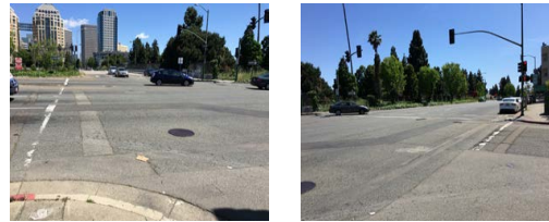
Exhibit C-13A: Prohibited Pedestrian Crossing on North and East Legs at Brush Street and 12th Street; Faded Crosswalk at Brush Street and 12th Street
