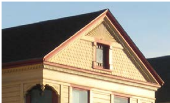
Attic windows, sunburst apices, fish-scaled shingles, dentils, and ornamental corner support brackets are character defining features of Queen Anne style residences in the District.
