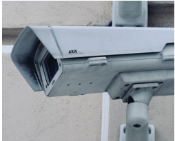
Install security cameras.
