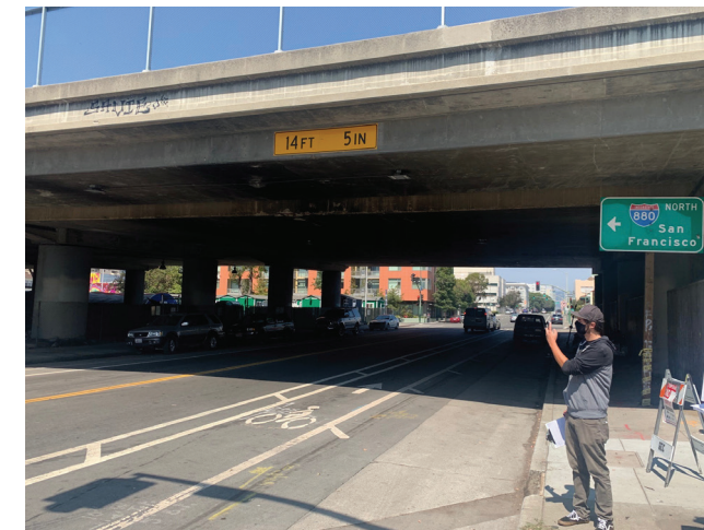
Example of poor vertical illumination
