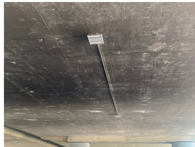
Typical existing LED luminaires
