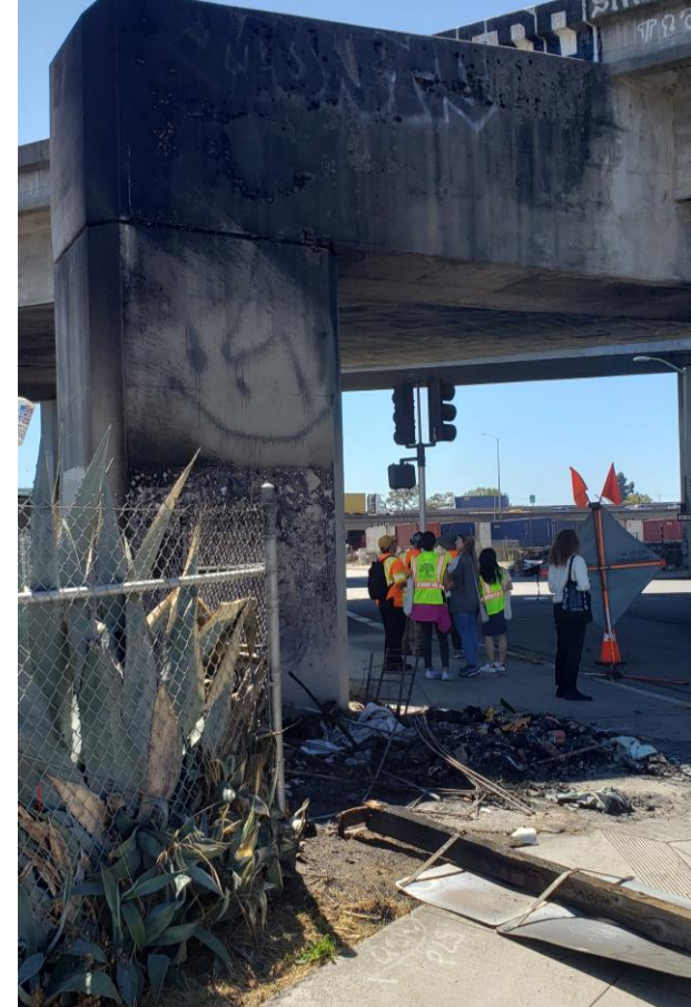
Debris from a fire near the 7 th Street undercrossing. Photo taken in August 2024.
