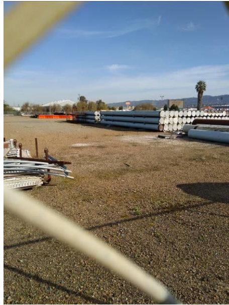
Photo #30 View of the pipe yard, located on the northeast corner of the site.
