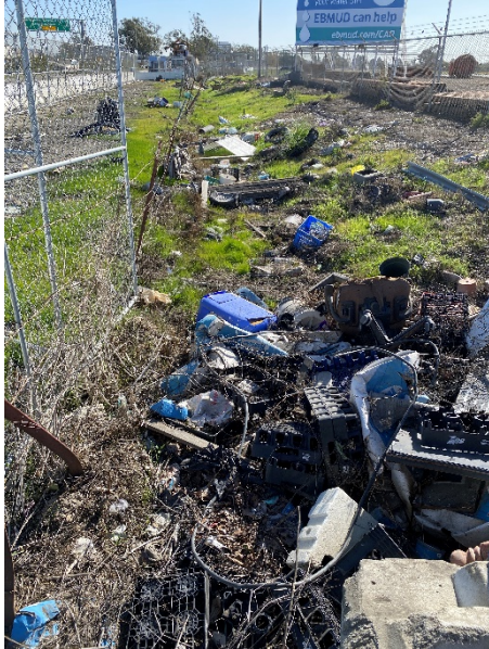
Photograph 1: Current conditions at Seasonal Wetland Ditch A, looking south from clogged culvert.
