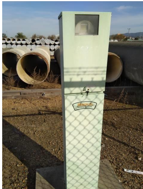
Photo #31 View of a power distribution meter, located in the pipe yard.
