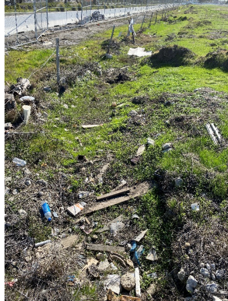
Photograph 2: Current Conditions at Seasonal Wetland Ditch B, looking south from clogged culvert. Location of Sample Points 1 and 2.
