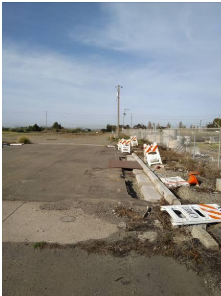
Photo #19 Additional view of the paved area, located on the northern portion of the site.
