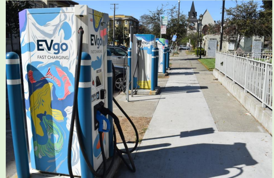
DC Fast Charger at Lafayette Square
