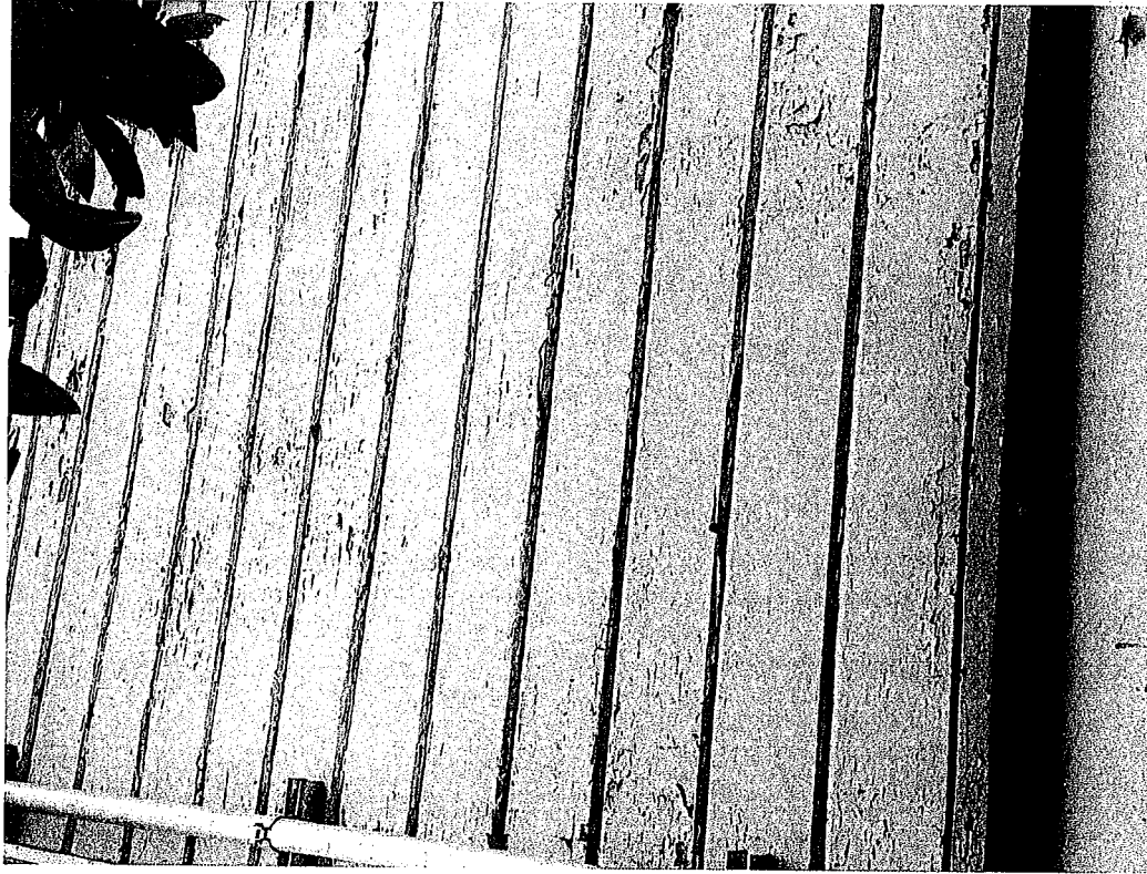
Image #3 An example of the exterior Siding to be scraped, sanded and painted (the whole house looks like this) Years 2017-2019 of the work plan
