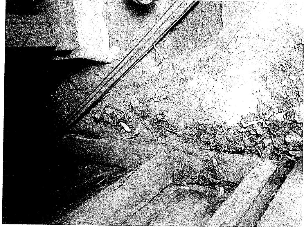
Image #6 Back addition foundation to be installed Years 2017-2019 of the work plan
