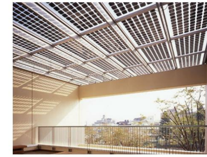
1 | Translucent Photovoltaic Panels
