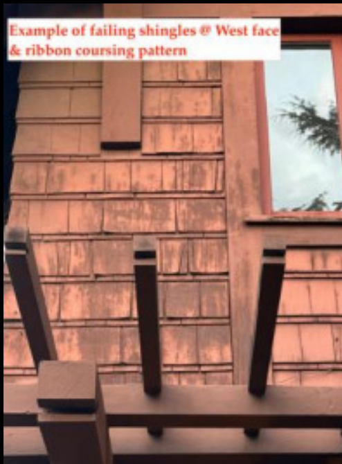
Failing siding. Split, missing portion. Making wall framing susceptible to rot
