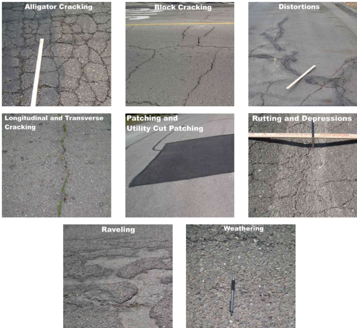
Figure 4: Asphalt Concrete Pavement Distresses
