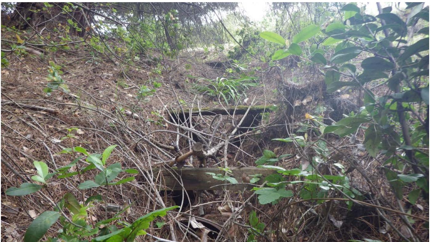
Site S3 (Feature F1). Wooden planks placed perpendicular to the ditch. View to the south.
