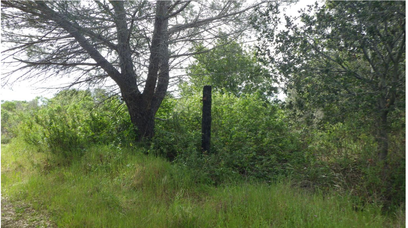
Site S1 (Feature F1). Overview of gate post. View to the west.
