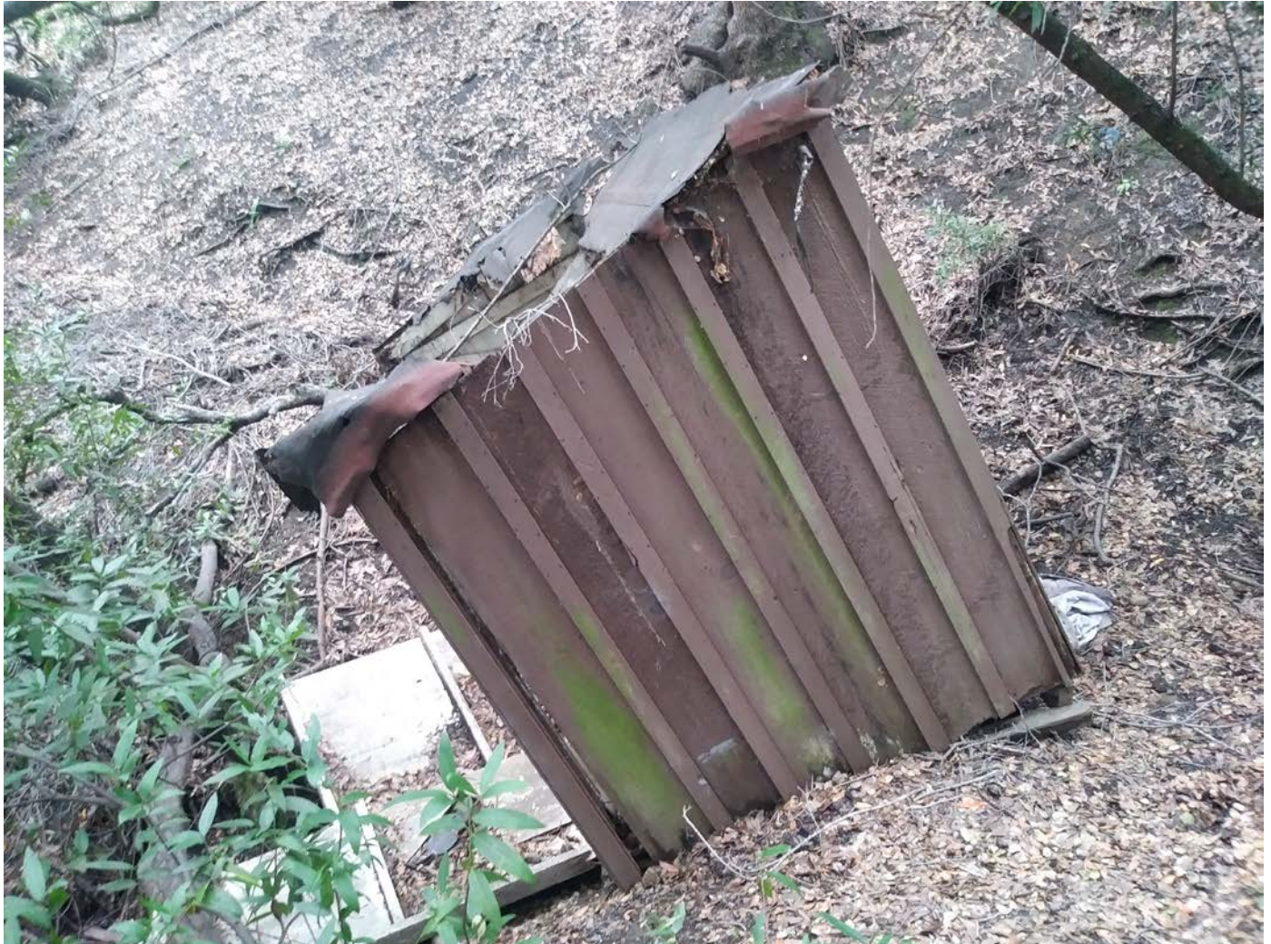
Site 7 (Feature F17a). Overview of board-and-batten sided latrine, the building is collapsing to the south into the canyon that it straddles. The south wall (left side) has completely separated and fallen to the south, downhill side of the latrine.
