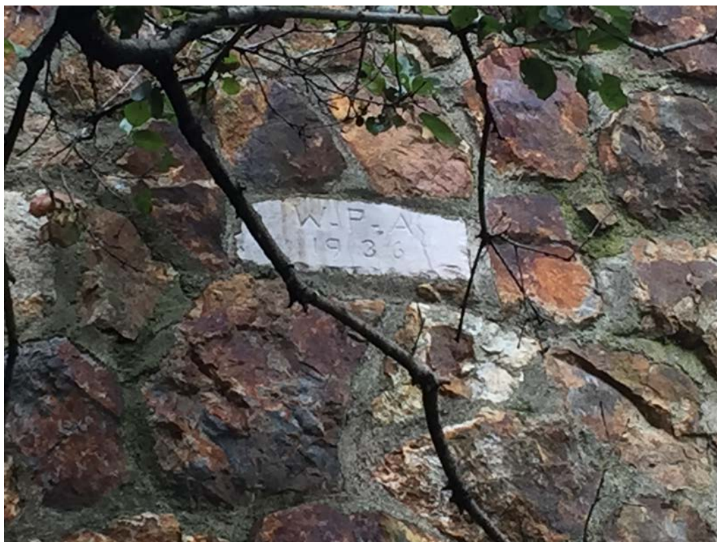
Site 7. Light-gray stone centered in chimney façade is incised "W.P.A. 1936." View to the north.
