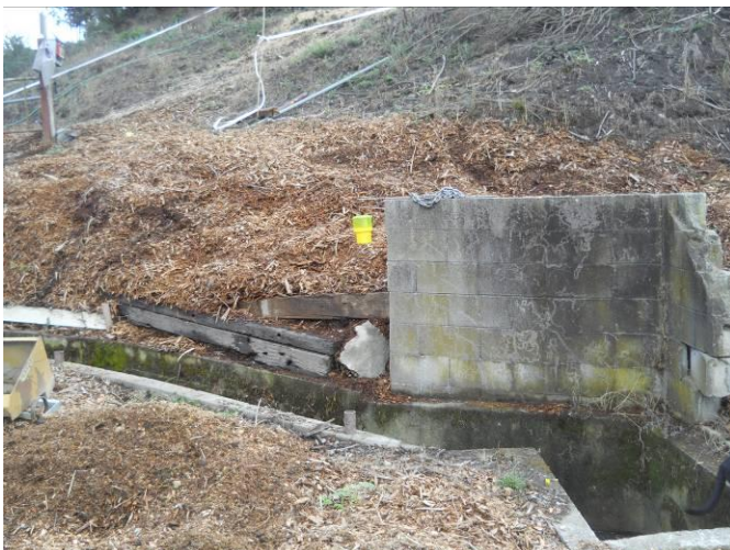
Skyline Ranch Water Conveyance Feature
