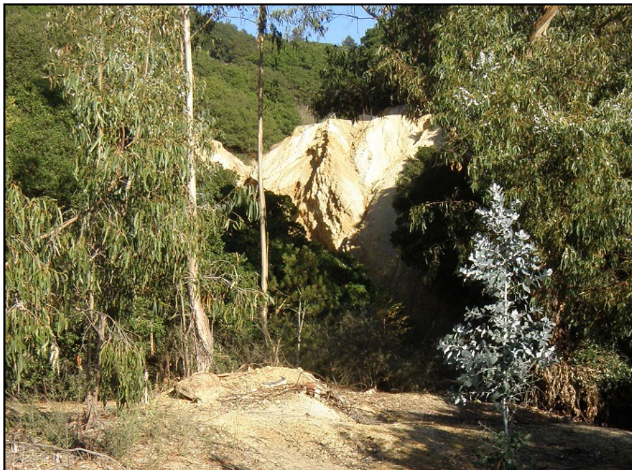
Upper tailings (above) with push pile of debris in foreground. View to East.
