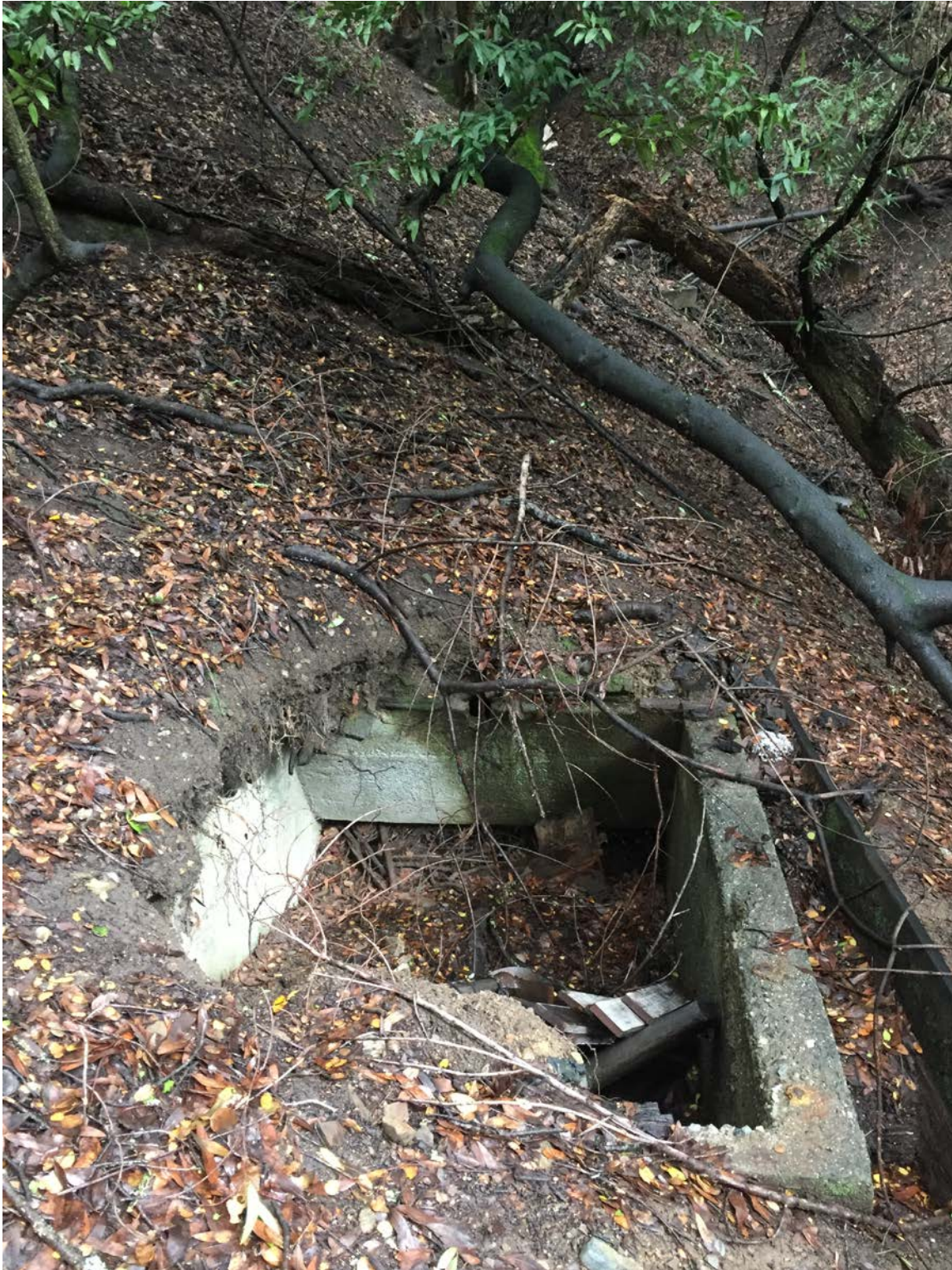
Site 7 (Feature F17b). Remnants of a wood-board top are visible on the west side walls of the concrete septic tank. Drain pipes from the latrine (Feature 17a) lead down the canyon and south to the septic tank. View to the east.
