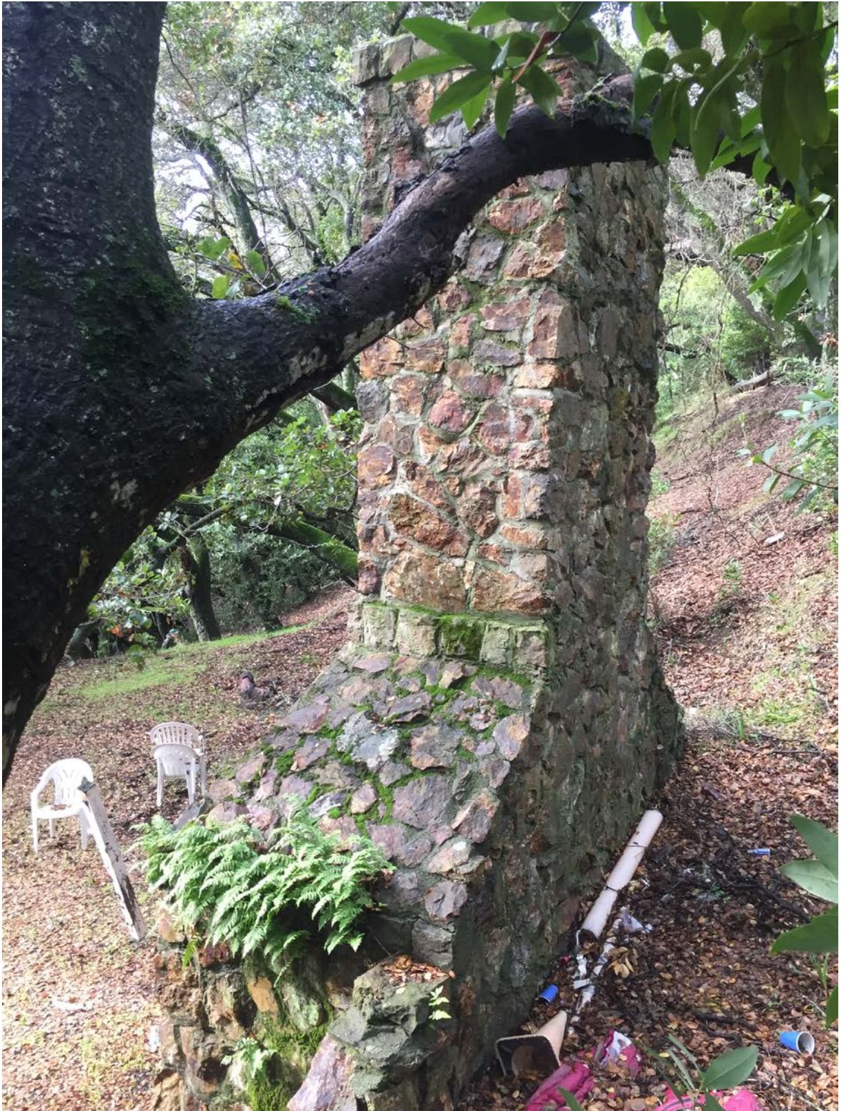
Site 7. View of the east elevation of the chimney, mortar joints are subject to deterioration from carbonic acid from moss, lichen, and ferns. View to the west-southwest.
