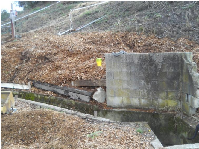
Skyline Ranch Water Conveyance Feature
