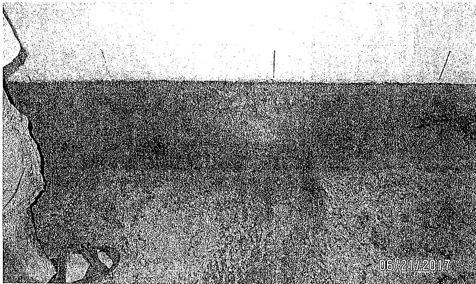
Photo 13, Beard v. Stewart, water stains
