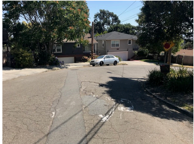
Figure 26: Parker Avenue Between Outlook Avenue East and West
