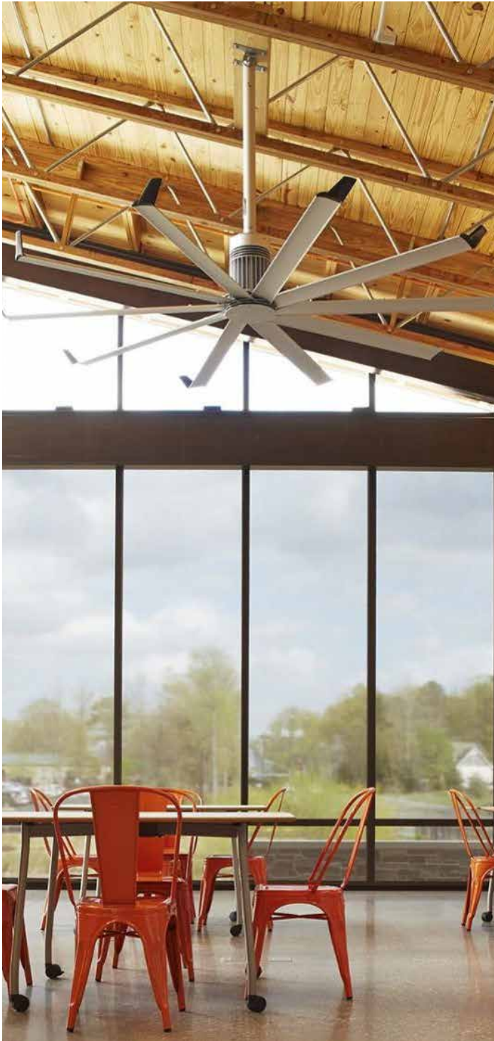
CEILING FANS PROVIDE AIR MOVEMENT THAT SIGNIFICANTLY IMPROVES THERMAL COMFORT.
