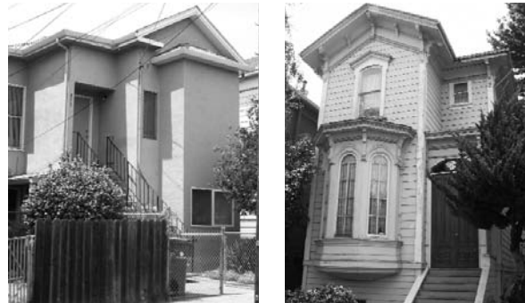
Some houses need help to recover from unwise modernization efforts; others need maintenance, paint, and wood restoration.
