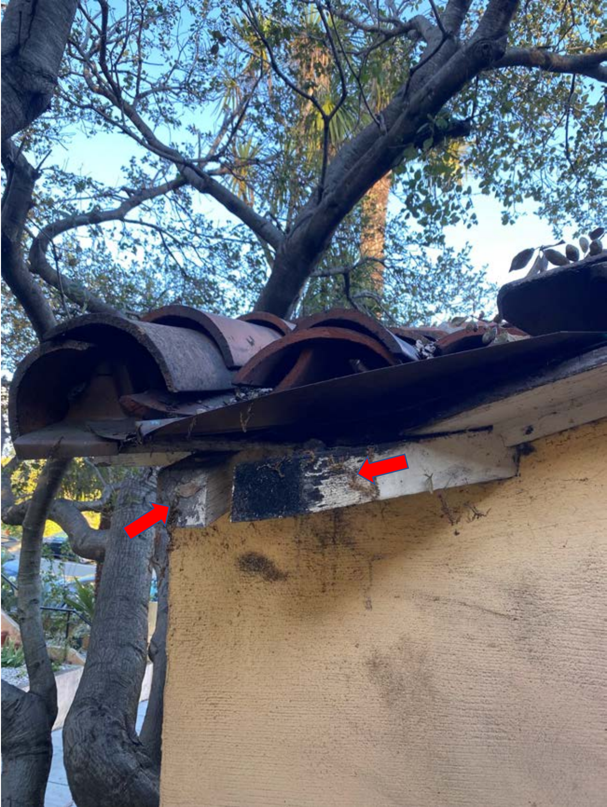
(Dry rot repair needed on multiple bungalow roof lines)
