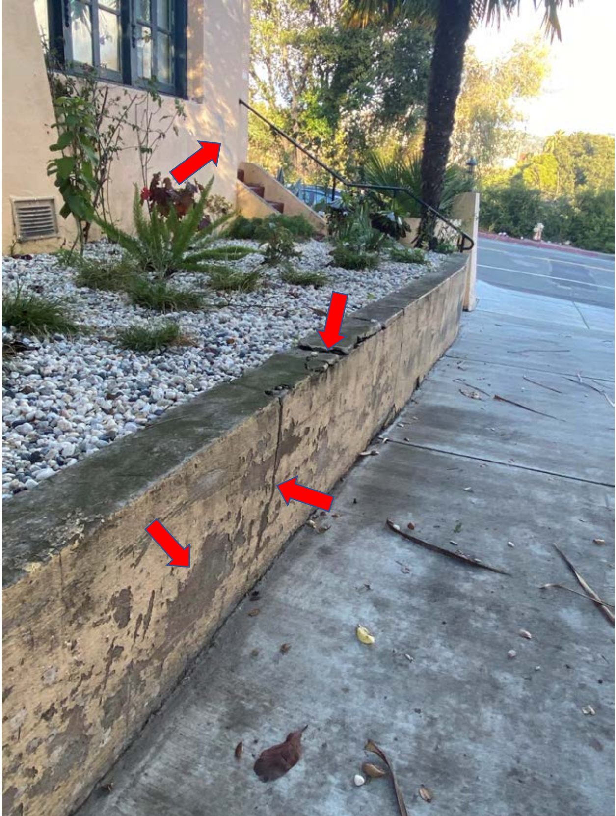
(Stucco damage on driveway retaining wall)
