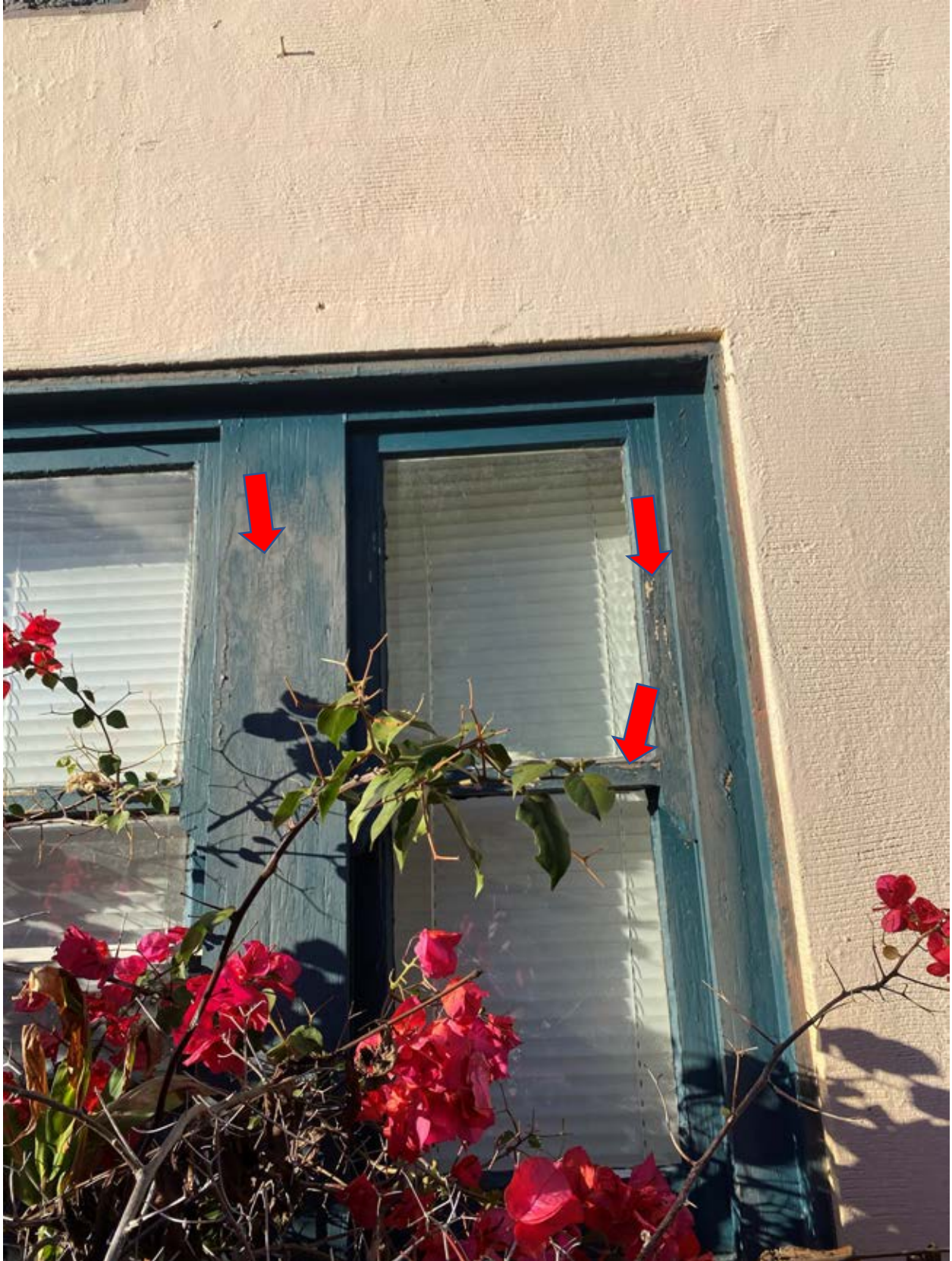
(Window framing containing dry rot and in need of restoration in kind to match original)
