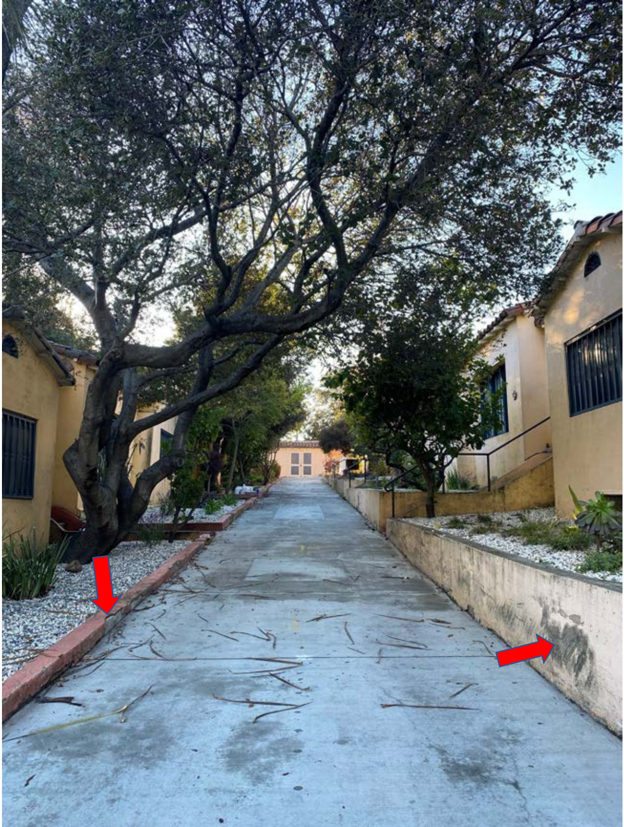
(Interior driveway walls heavily damaged, stucco, paint and cement)
