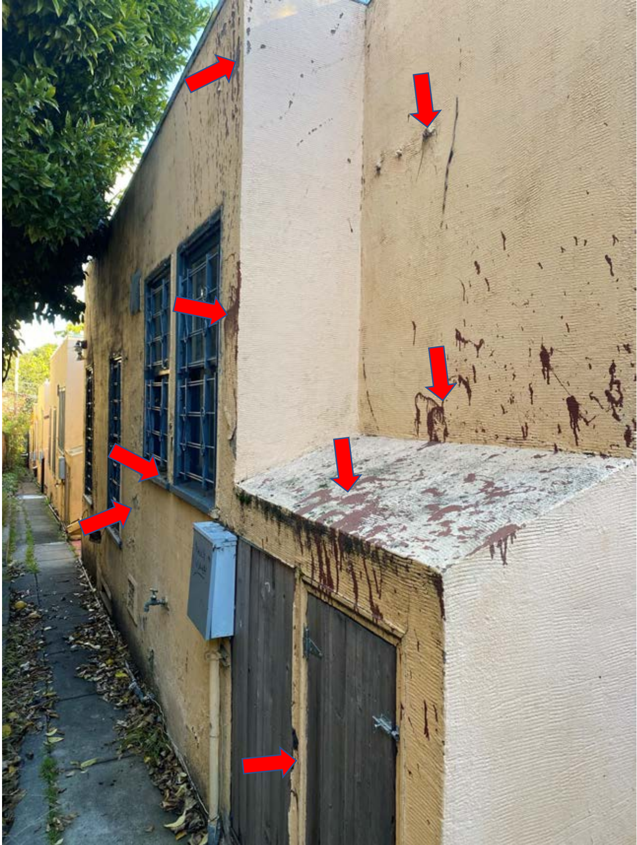
(Damaged stucco siding, paint spillage and cracking)
