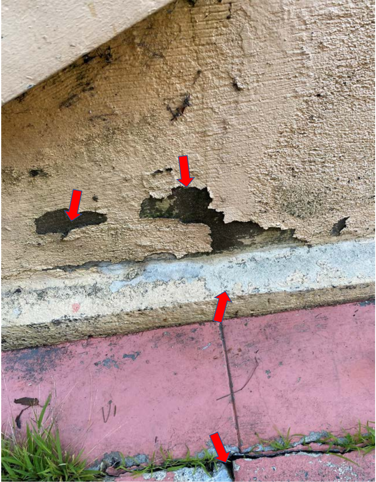
(Damaged walkway and stucco siding)
