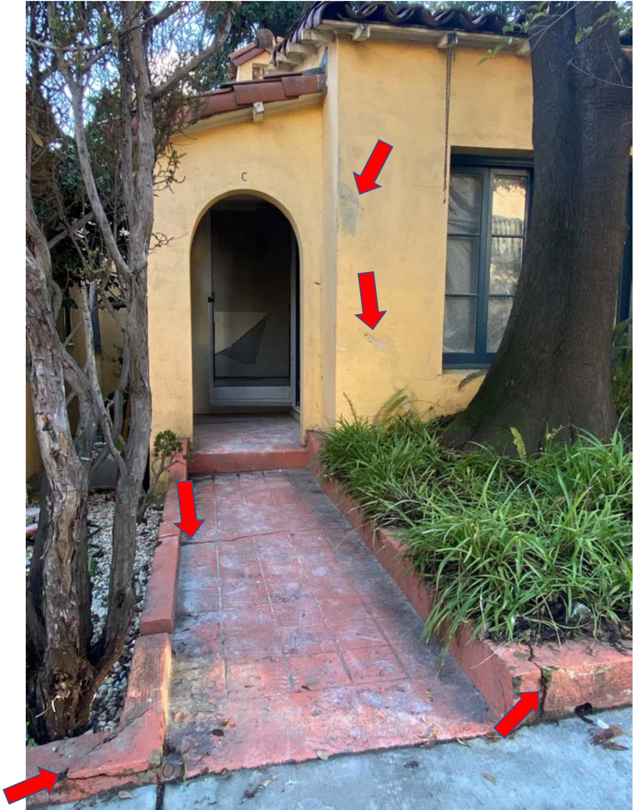
(Concrete damage on walkway entrance to bungalow)
