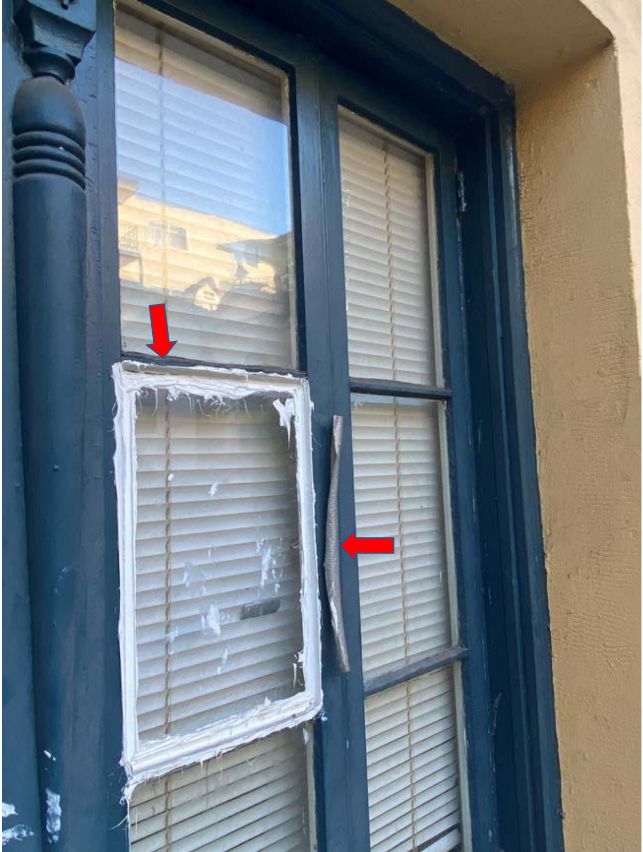
(Improper caulking and repair. Needs replacement/restoration) in kind, to match original
