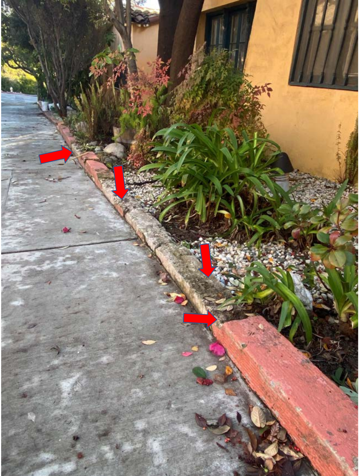
(Driveway landscaping wall damage. Broken pieces and concrete damage)
