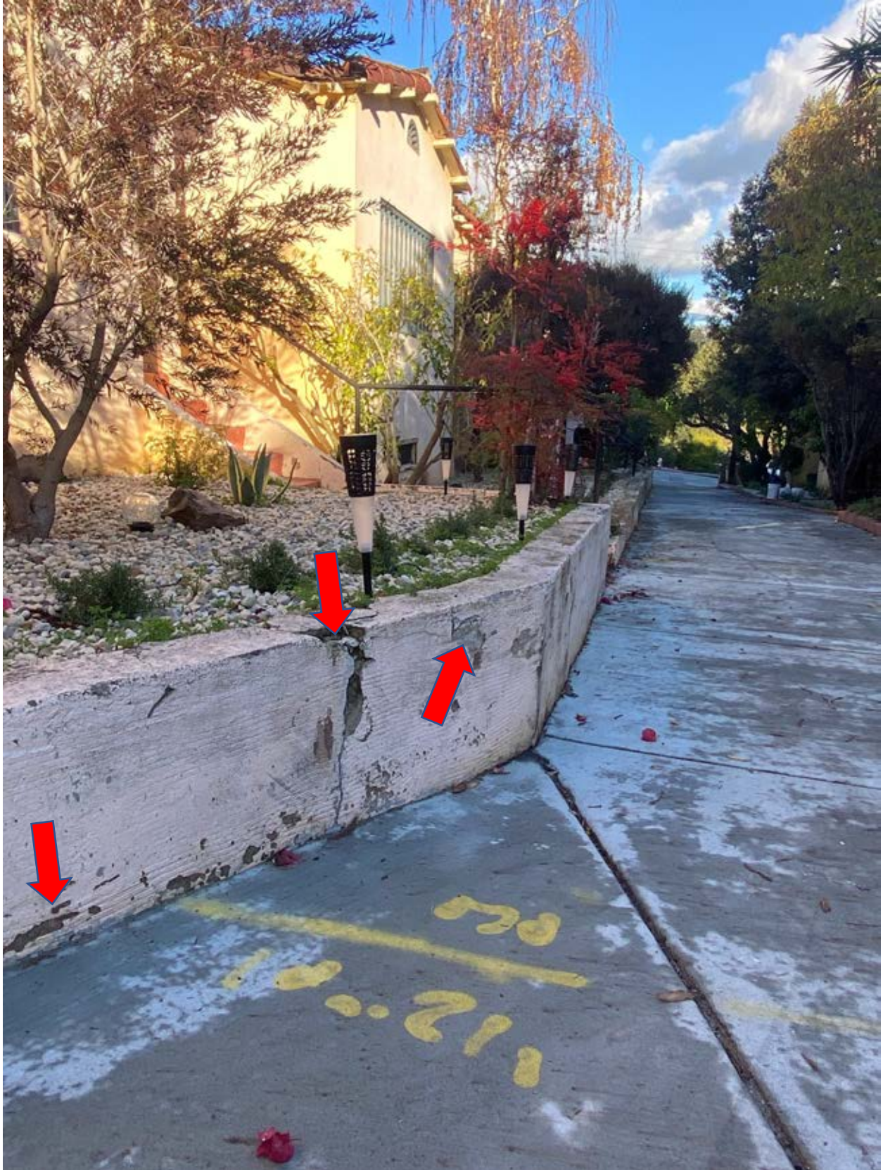
(Additional driveway retaining wall damage)
