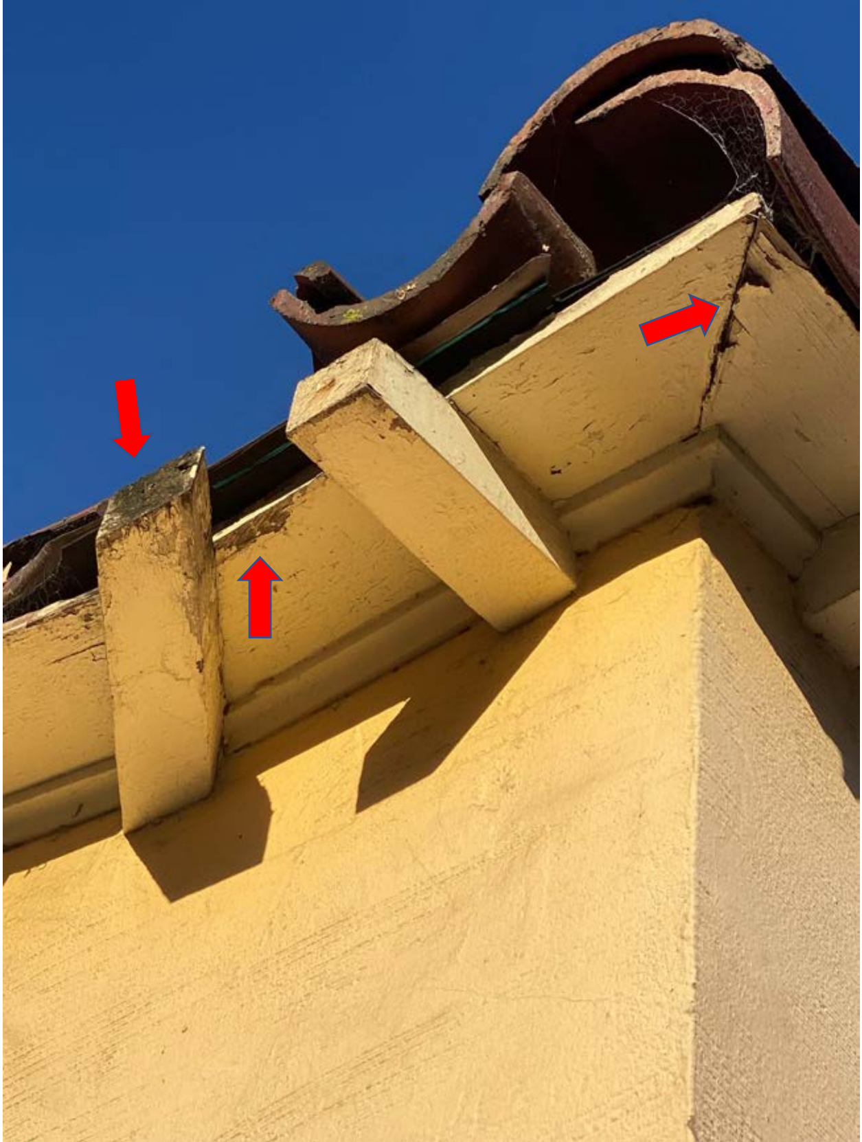
(Additional roofline dry rot)
