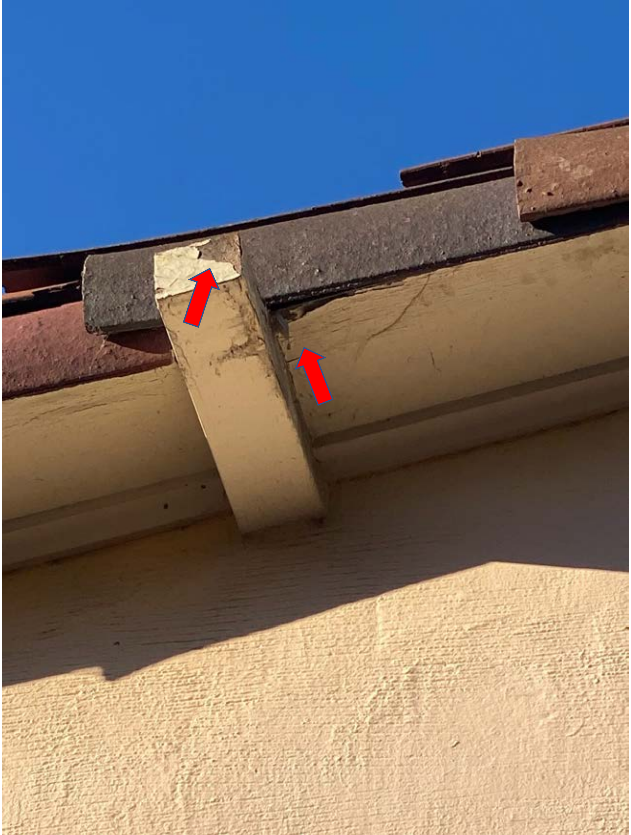
(Roofline dry rot on multiple bungalows)
