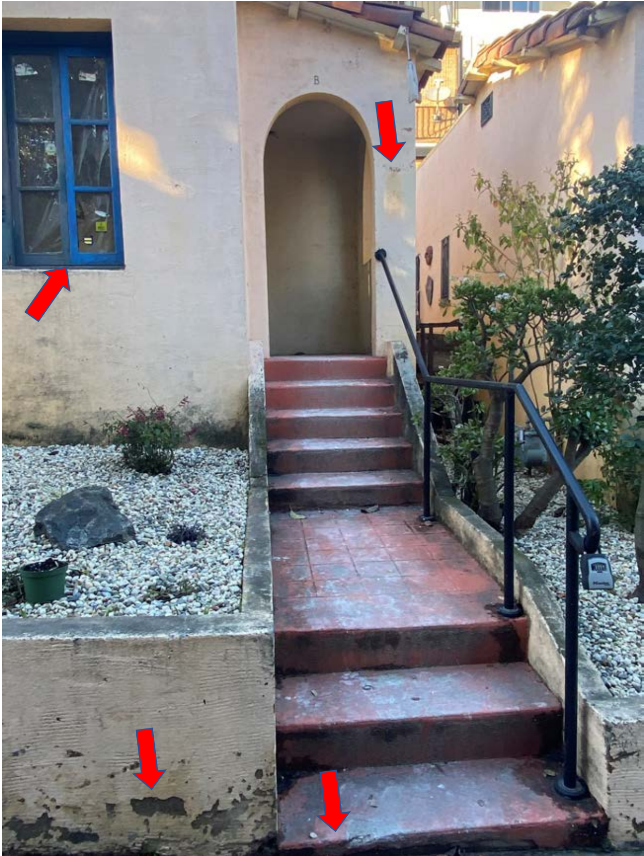
(Mismatch paint on windowsills, damage to stucco and concrete at bungalow entrance)
