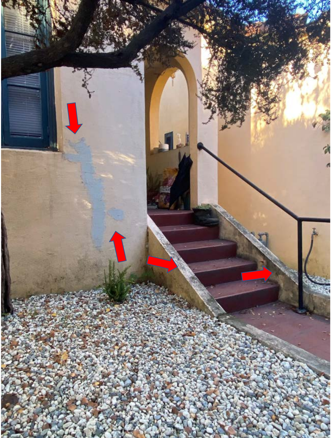
(Improper repairs to prior stucco damage. Retaining wall restoration needed)
