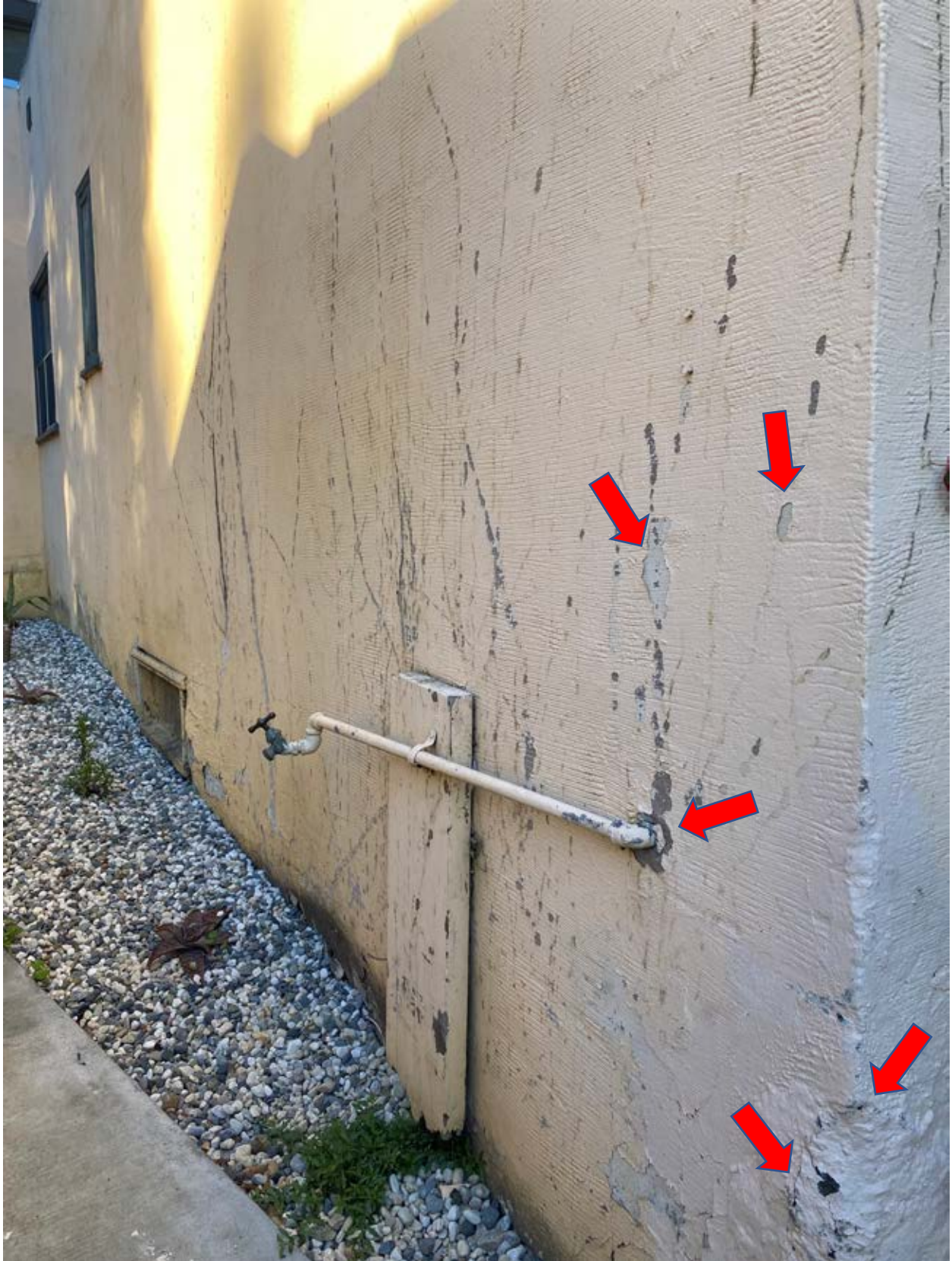
(Damaged Stucco siding)
