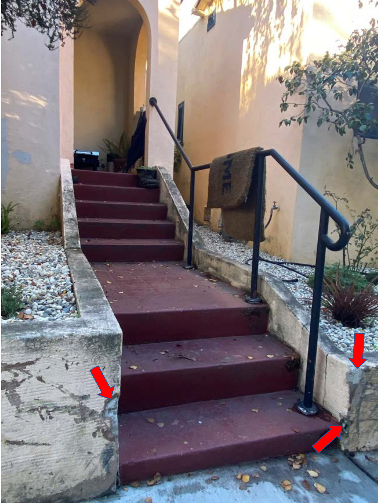
(Damage and cracking on bungalow entrance way)
