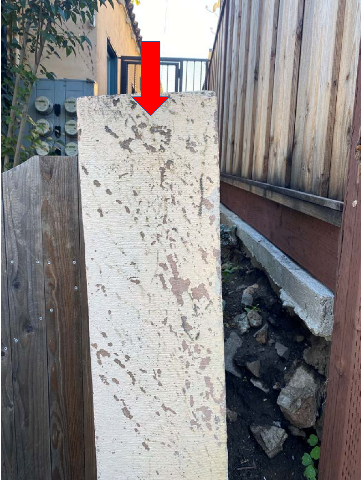
(Street facing wall with extensive paint/stucco damage)
