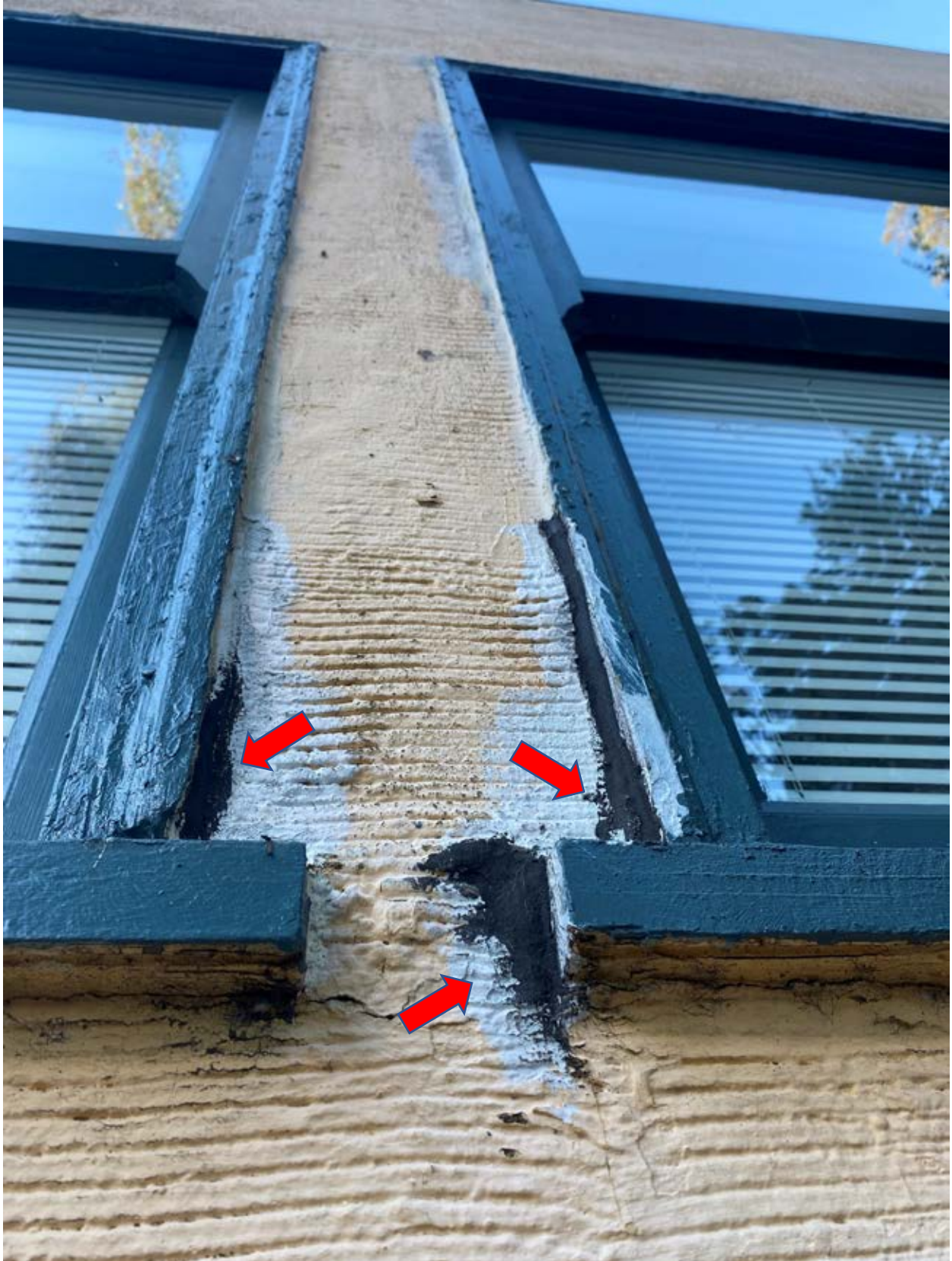
(Improper caulking and repair work on windowsill. Needs restoration)
