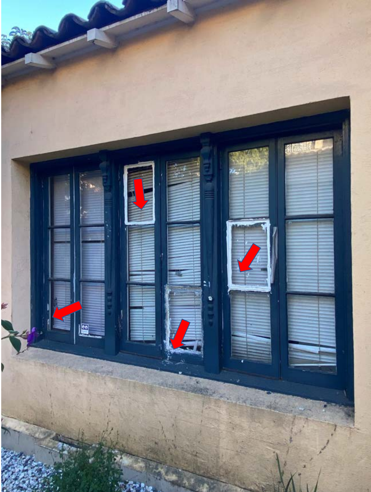
(Additional improper caulking/repairs)
