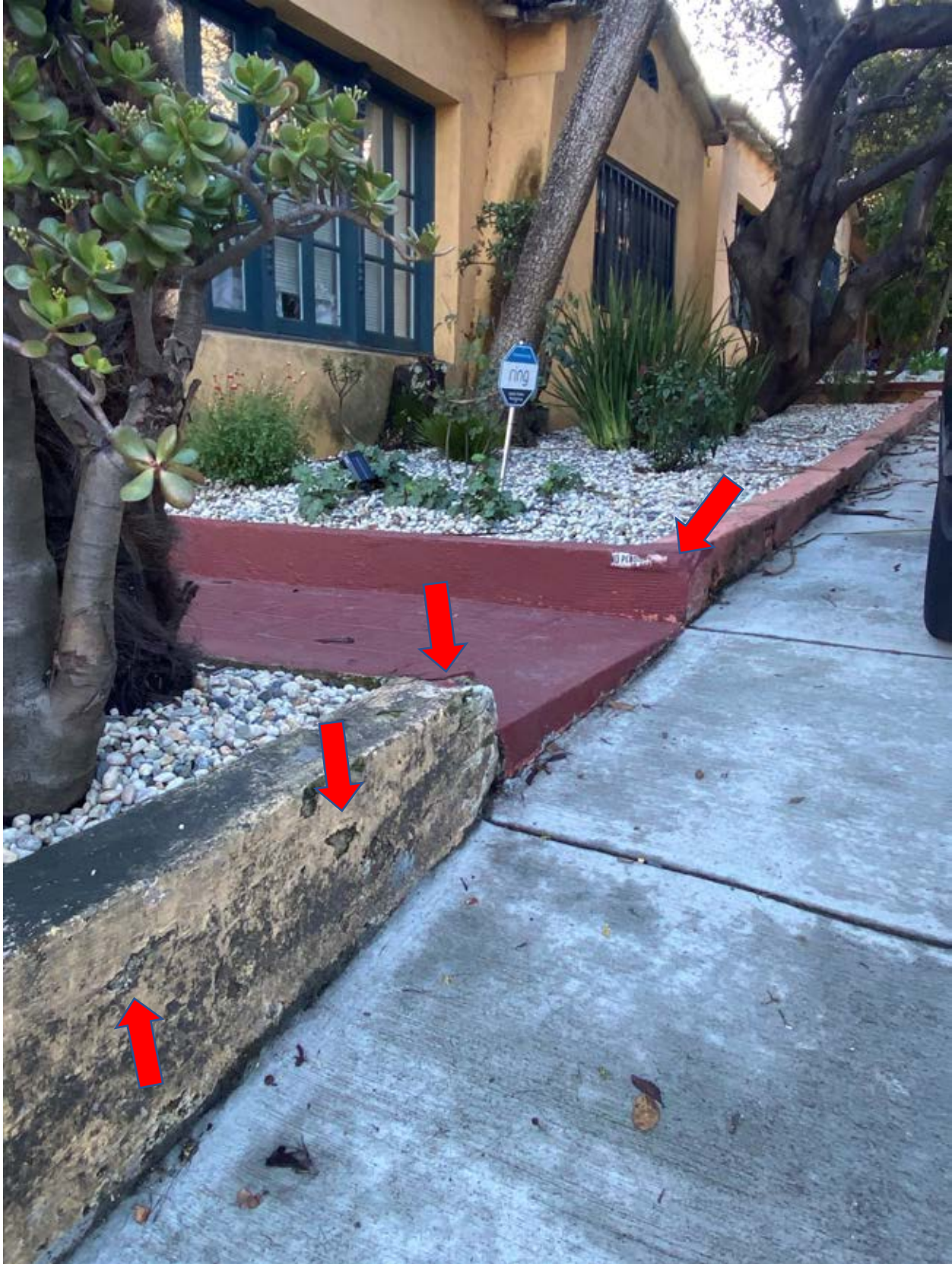
(Stucco damage and mismatched paint on walkway)
