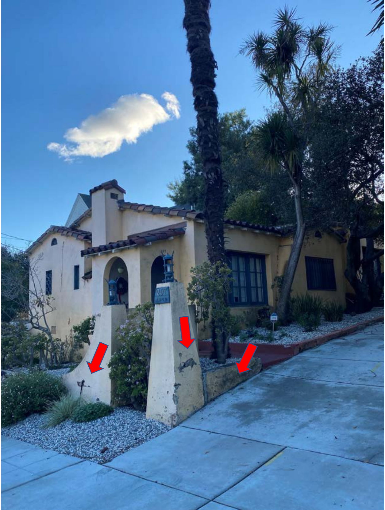
(Front entrance damage, cracking and stucco repair)
