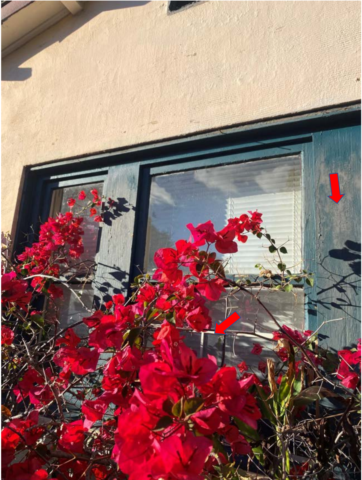
(Windowsill paint cracking)
