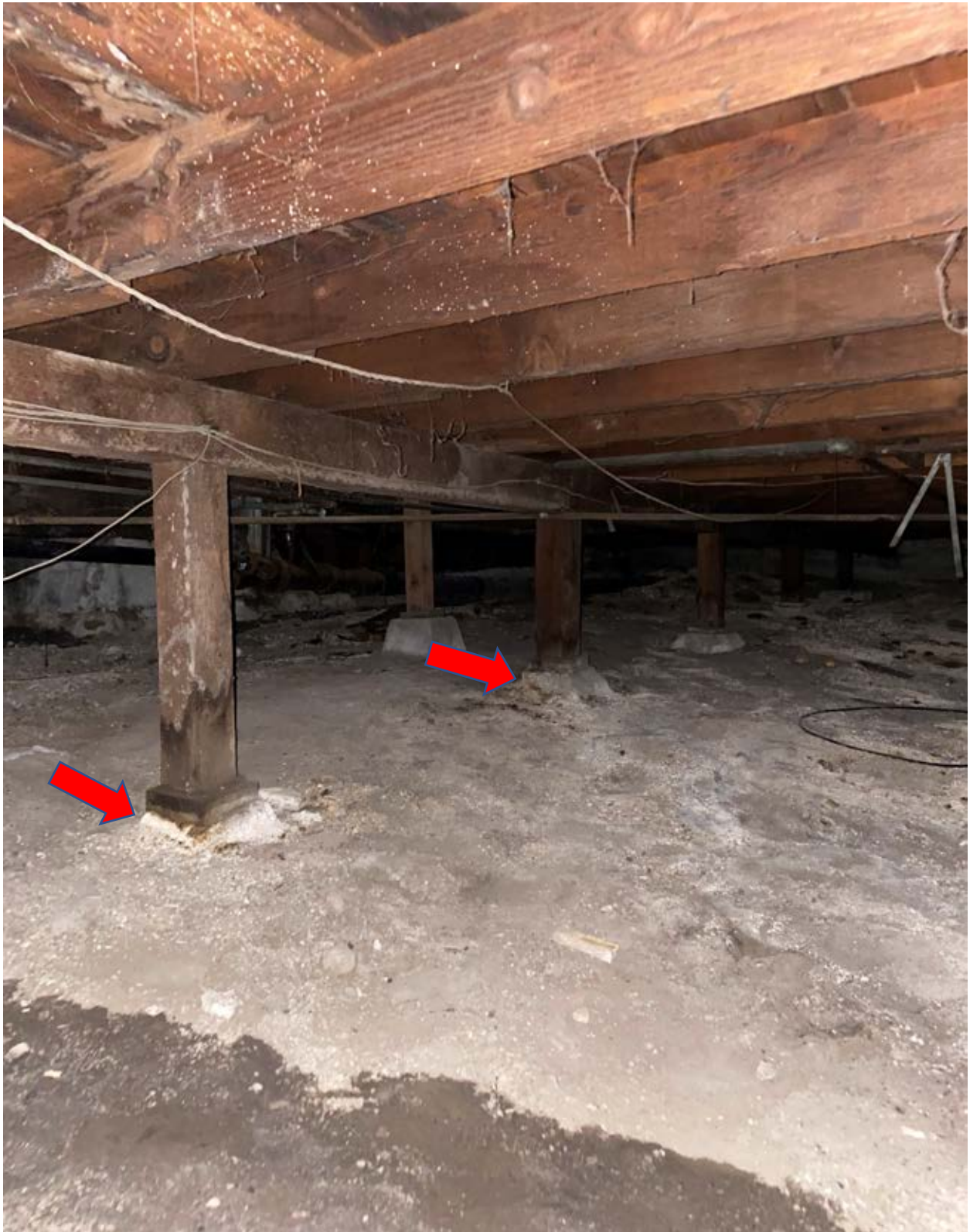
(Soft-story structural/seismic issues that need to be reinforced)
