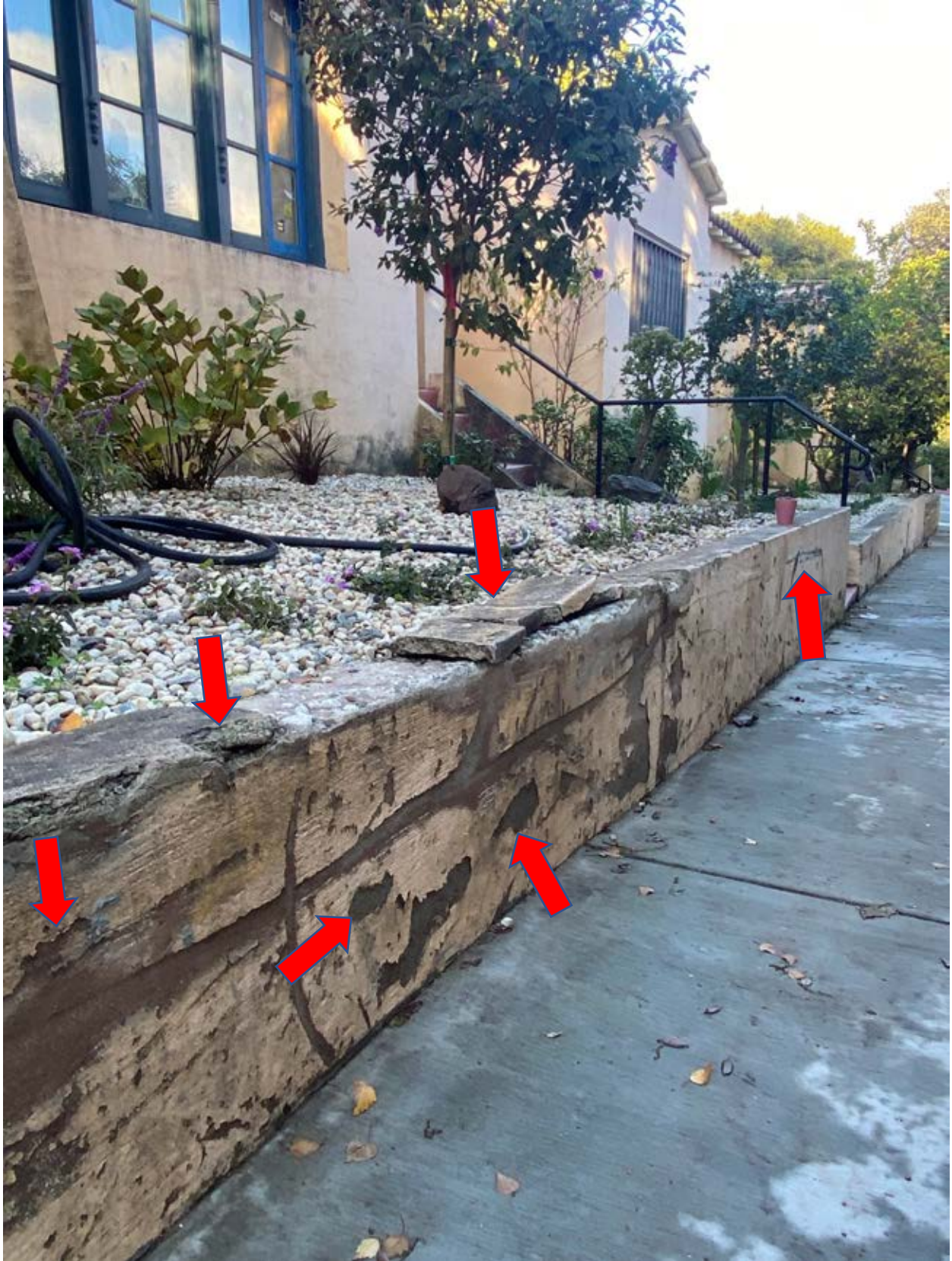
(Major damage on portion of driveway retaining wall. Stucco damage and broken cement)
