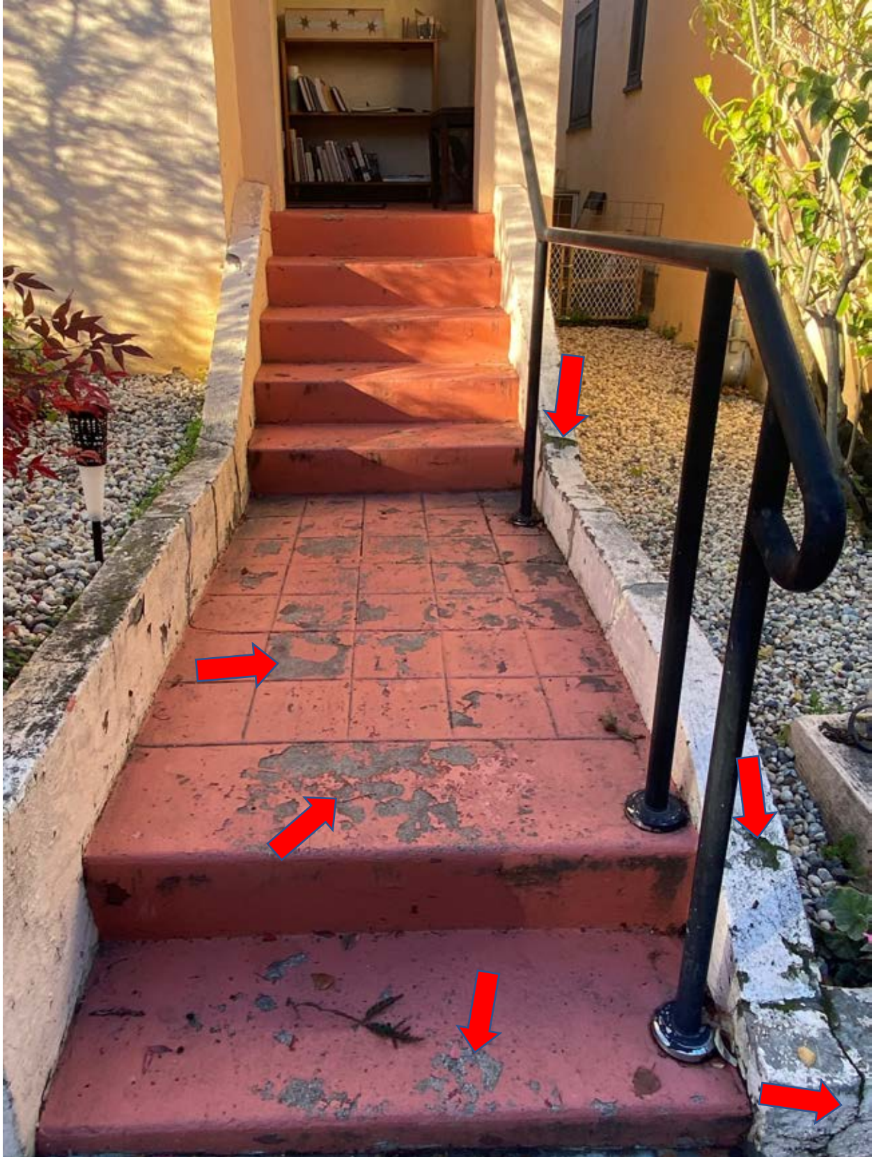
(Paint peeling and damage on bungalow walkway. Stucco cracking and damage on retaining walls)
