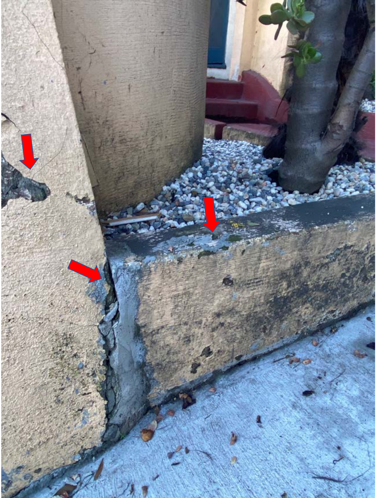
(Major cracking and improper repairs on driveway portion of entrance post)
