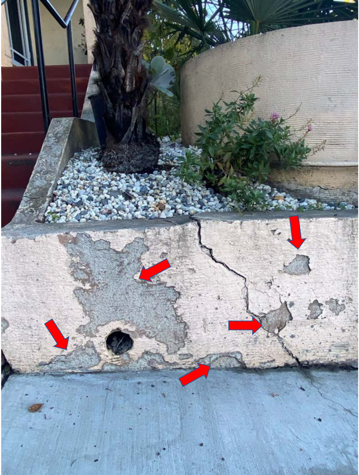
(Major cracking and stucco damage on driveway retaining wall)
