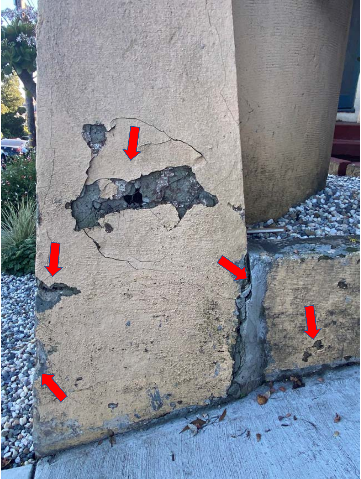
(Major cracking on and stucco damage on street facing entrance posts)
