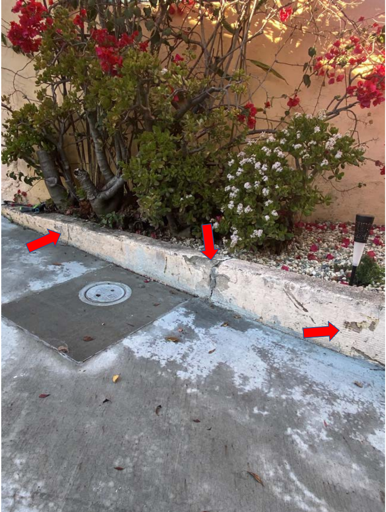
(Driveway retaining wall cracking, settling, stucco damage. Needs repair/replacement)
