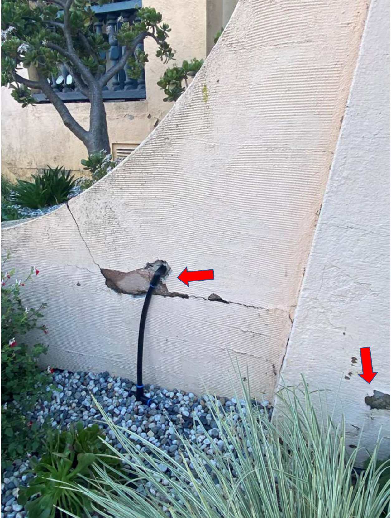
(Improper repairs to street facing walls)
