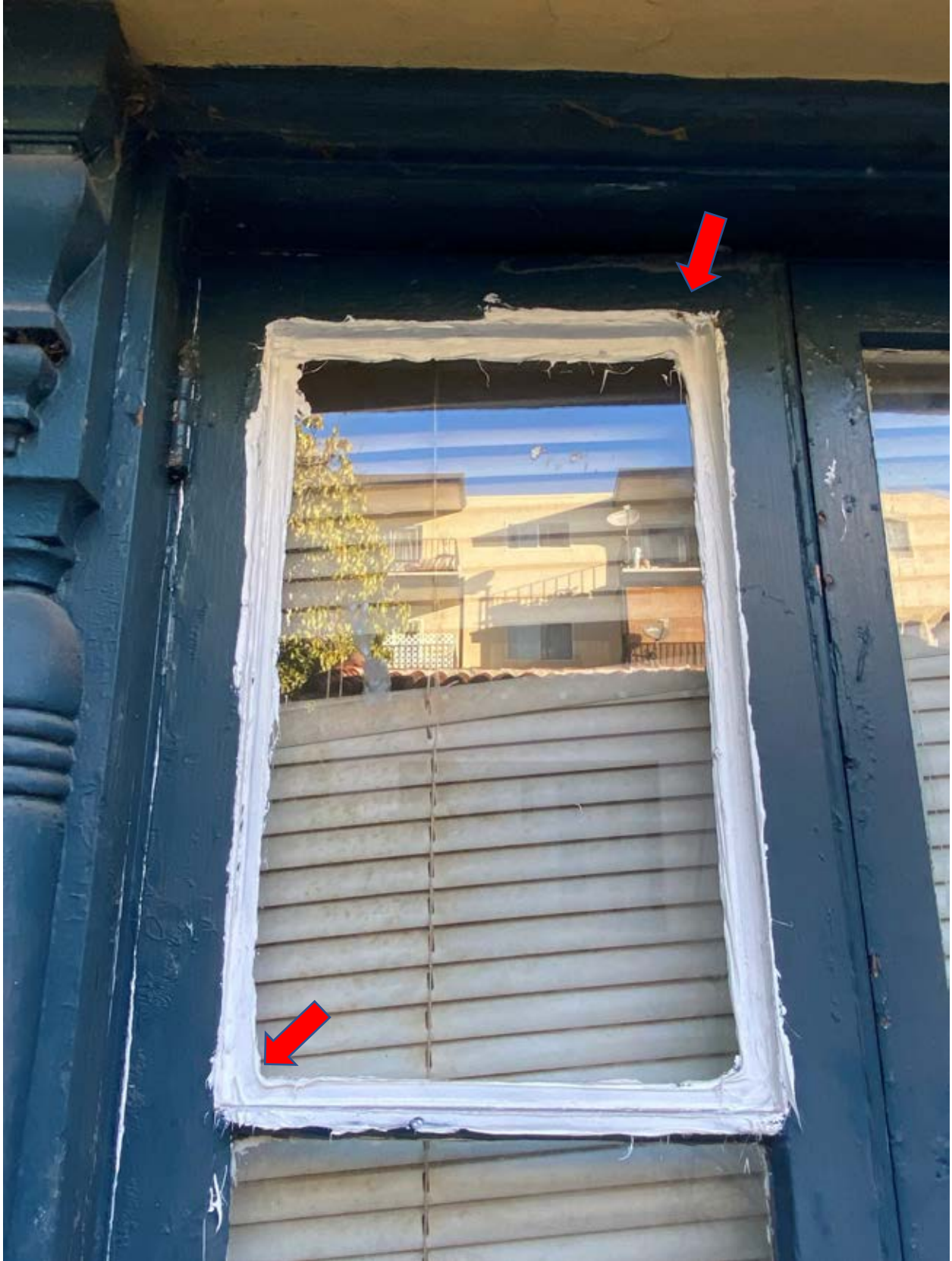
(Example of improper caulking/repairs from prior deferred maintenance)
