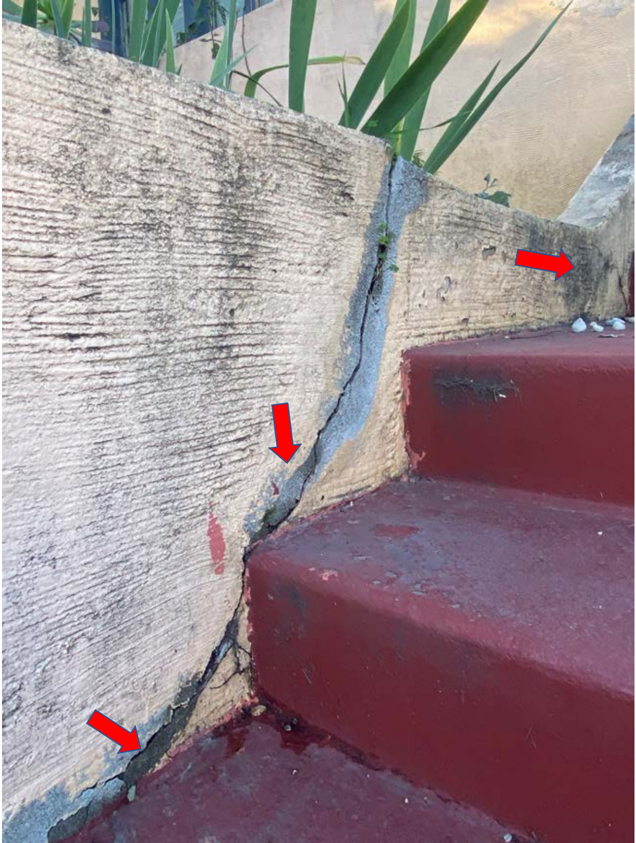
(Cracking and improper stucco repair on bungalow front entrance)
