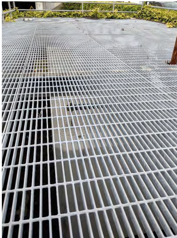
Photograph 14 – ConVault AST located in parking lot at Site 2, covered with metal grating and surrounded by fencing.
