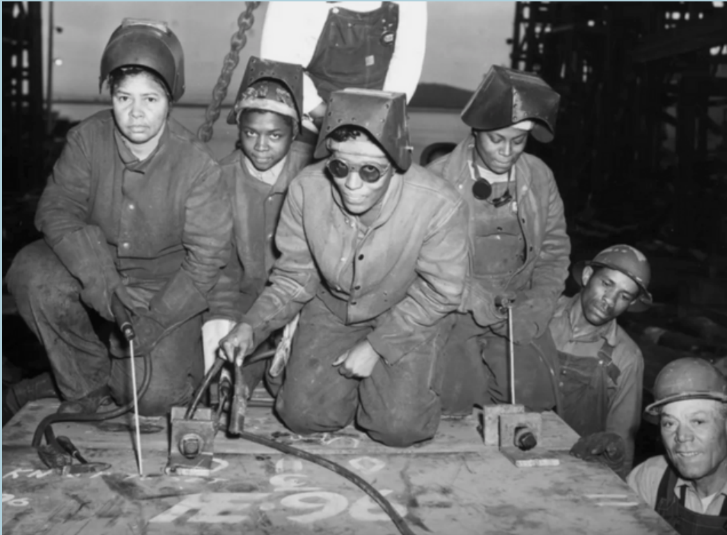
Welders prepare to work on SS George Washington Carver in Richmond, California, 1943. E. F. Joseph/Anthony Potter Collection/Getty Images
