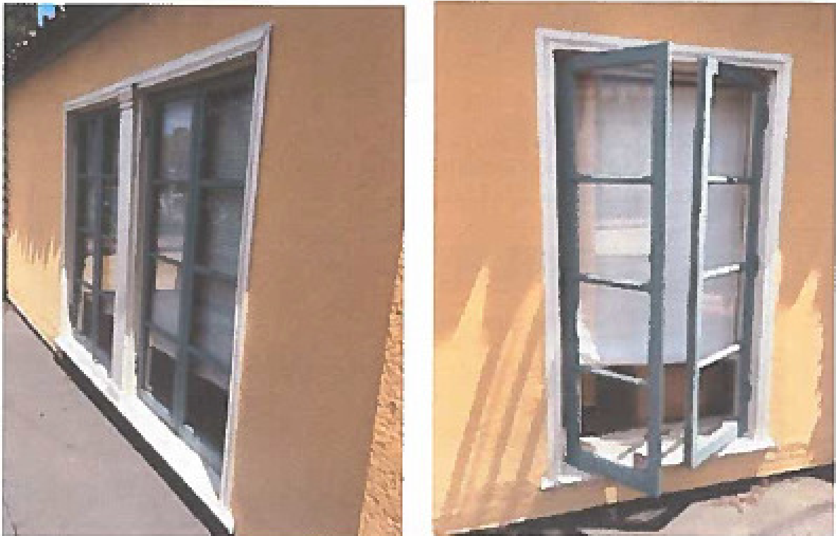
Figure 1. a. Windows right side, second floor toward street. Note the square column decoration between the double windows, which will be preserved. b. Window right side second floor toward rear of house
