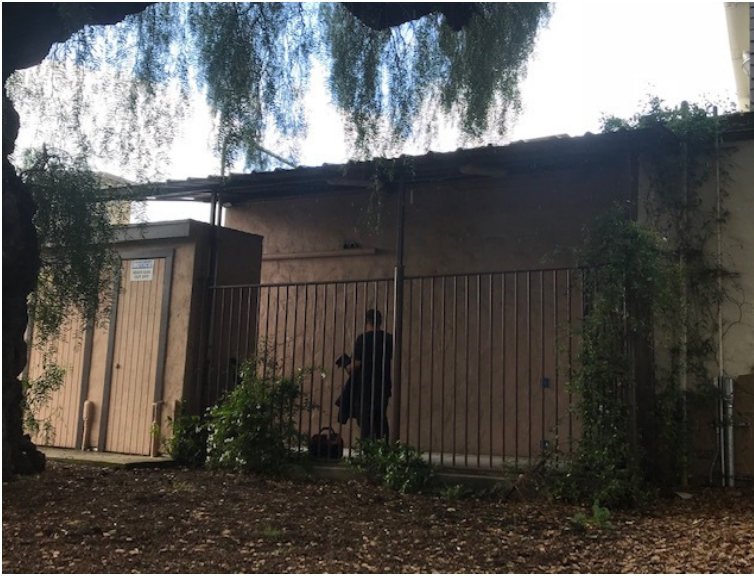
Repaint rear entrance area to match existing structure (correct error made by dispensary operators)
