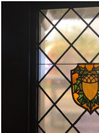
Replace missing piece
