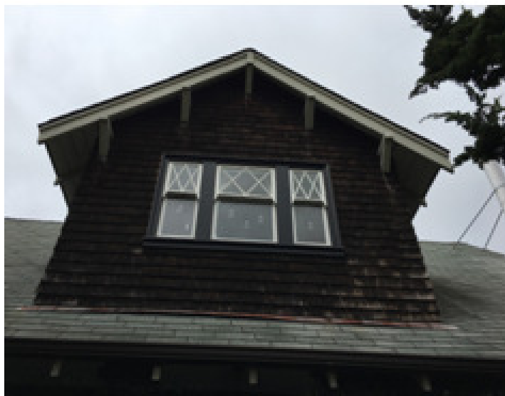
#2: replace windows in gable #3: replace gable dormer shingles
