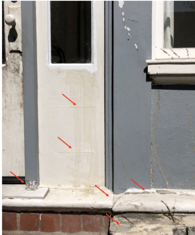
ROTTING AT MUDSILL TRIM, DOOR THRESHOLD AND SIDELITE PANELS, NON- CLINKER BRICK INSTALL, CORRECT WATERPROOFING
