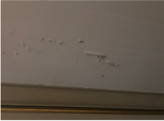
Left: Close-up of water stains.
