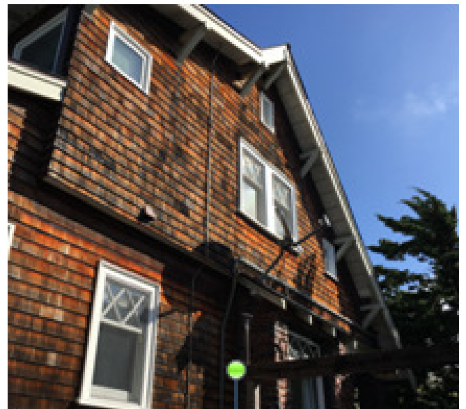
#5: clean/repair/replace shingles & window trim at rear & sides
