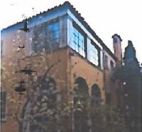
Figure 5. The three double second story windows on the left side and rear of the house, will be replaced during the third phase, retaining the original square column detail, window design and hardware.
