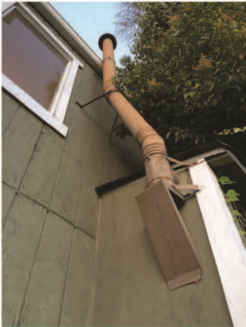
ROT ON T-111 SIDING
