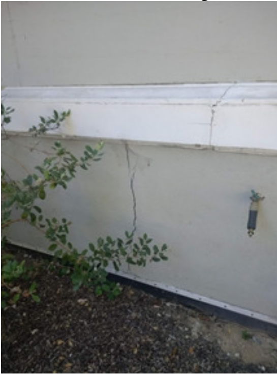
#1: Cracking walls west side
