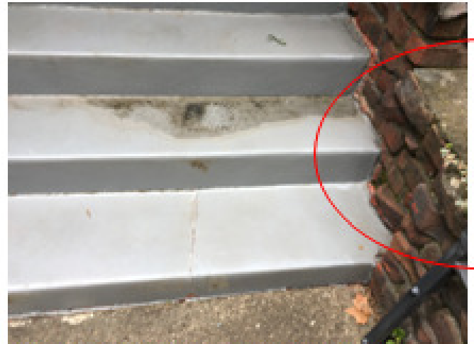
#4: repair/replace cracked front steps
