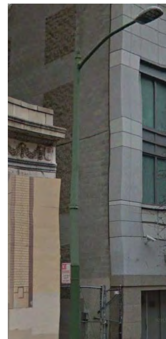
EXISTING 11TH AND 12TH STREET LIGHT - TO BE REPAINTED
