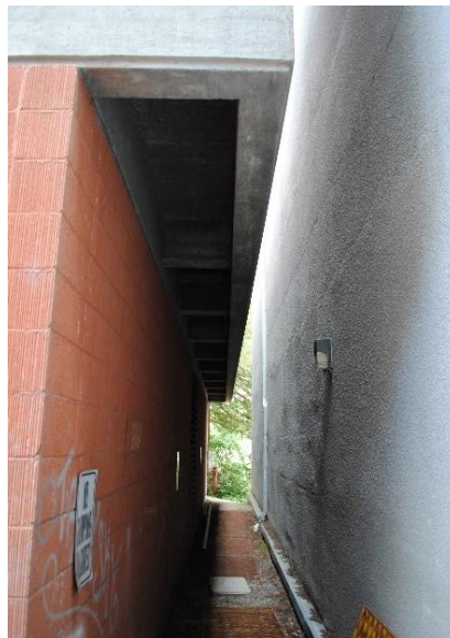
Figure 110. North façade of the Ceramic Arts Center (left), several feet from the Oliver & Ralls Building (right), looking west.
