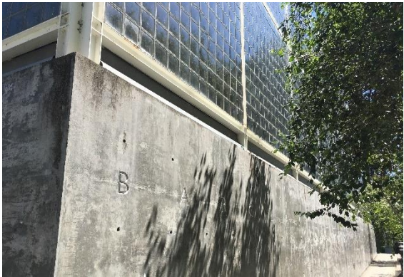
Figure 138. Polished concrete base with exposed concrete formwork tie-holes and incised, silver-painted lettering, looking southeast.
