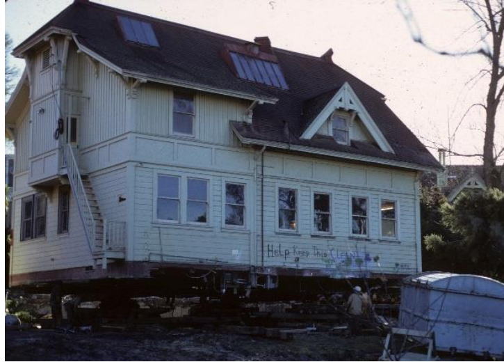
Figure 24. West and north facades of the Carriage House raised up on temporary foundation for relocation, 1973. Source: CCA Libraries Special Collections.
