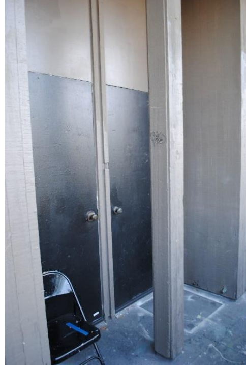
Figure 69. Typical recessed entrance with two tall metal doors, located on the second story primary façade.
