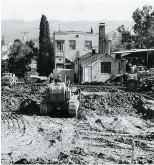
Figure 48. South façade of B Building during site clearing and construction of the Noni Eccles Treadwell Ceramic Arts Center, 1973. Source: CCA Libraries Special Collections.
