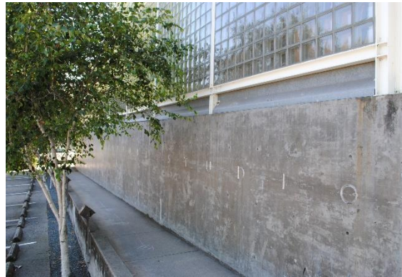
Figure 139. Galvanized metal louvers above the concrete base, within the steel grid frame, looking northeast.
