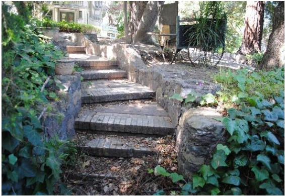
Figure 165. Staircase paved with Carnegie bricks, flanked by masonry retaining walls with ceramic pots.
