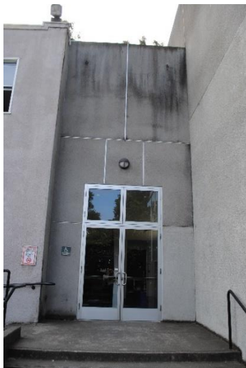
Figure 132. Hyphen volume with ADA-accessible entrance at the north end of the west façade of the Oliver & Ralls Building, abutting the B Building (left), looking east.
