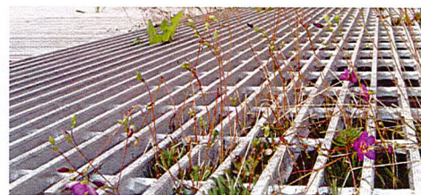
METAL GRATE LID AT BIORETENTION BASIN
