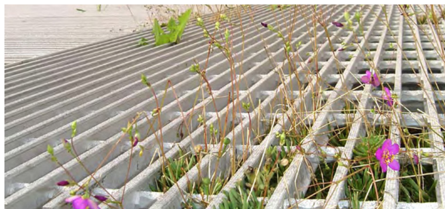
METAL GRATE LID AT BIORETENTION BASIN
