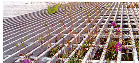
METAL GRATE LID AT BIORETENTION BASIN
