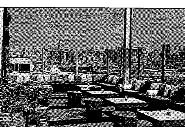
3 GLASS GUARDRAIL AT ROOF DECK
