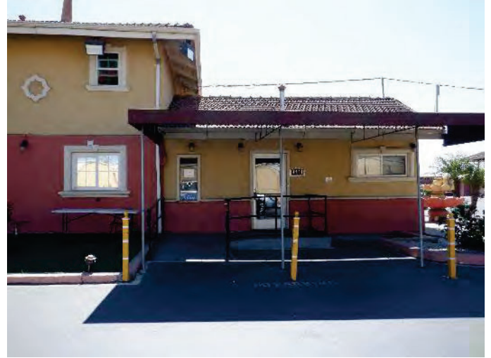
Photograph 3: East building showing office entry facing the driveway. Camera facing south. August 31, 2022.
