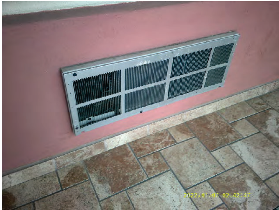
11. Guest room heat and AC unit
