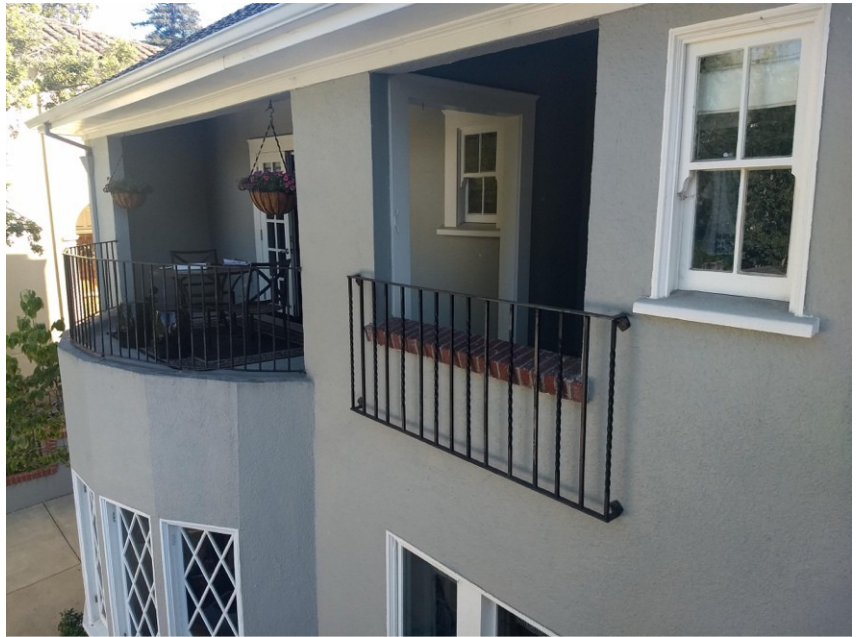
Figure 6. 676 Longridge Road, detail of rear (north) elevation showing recessed area of second floor level, view facing southeast.
