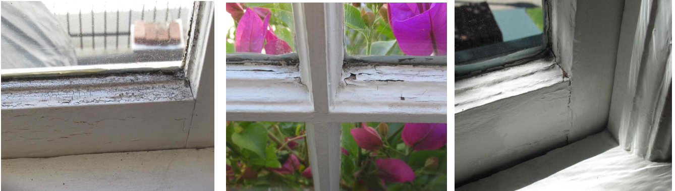
Samples of the many window frames whose wood is dried out, stained in places, with damaged paint.
