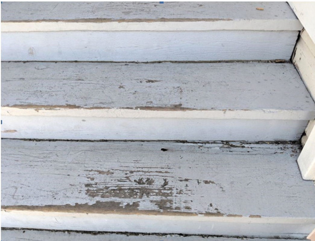
Dry rotted treads on the front staircase.
