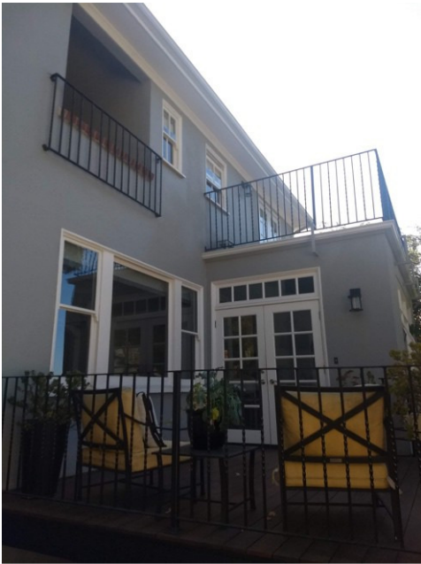
Figure 5. 676 Longridge Road, detail of rear (north) elevation showing kitchen volume, view facing southwest.
