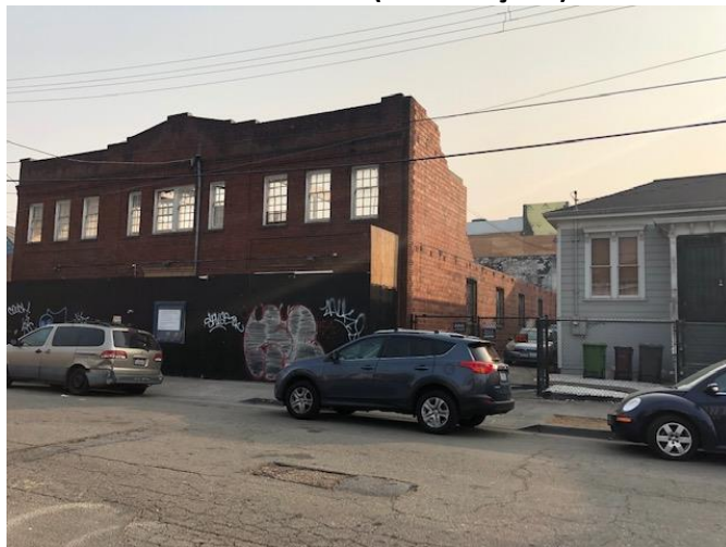
671 24th St north elevation, camera facing south-east – brick and tile shell after fire
