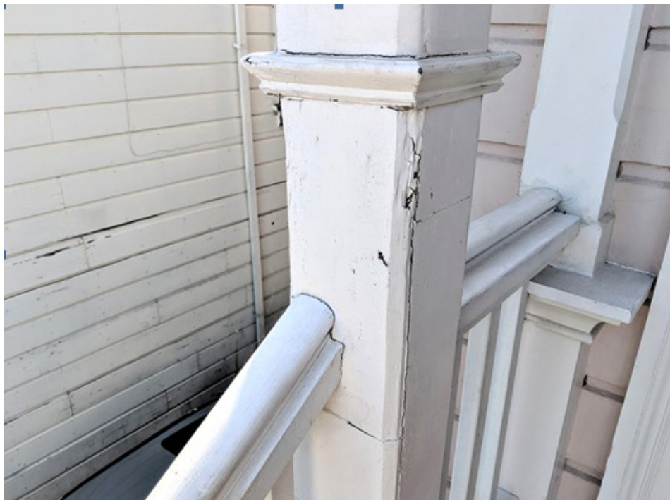
Patched dry rotted square chamfered columns located on the portico porch. They should be replaced with historically accurate turned balustrades.
