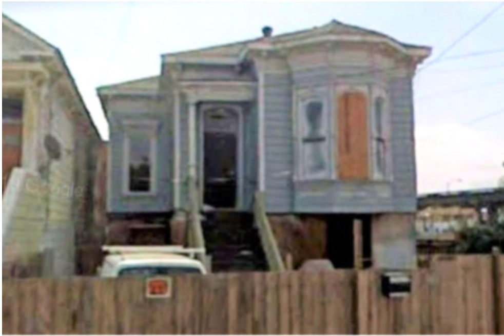
(2010) The Martin House during initial renovation, after all stucco was removed and the house was lifted 2.5'.
