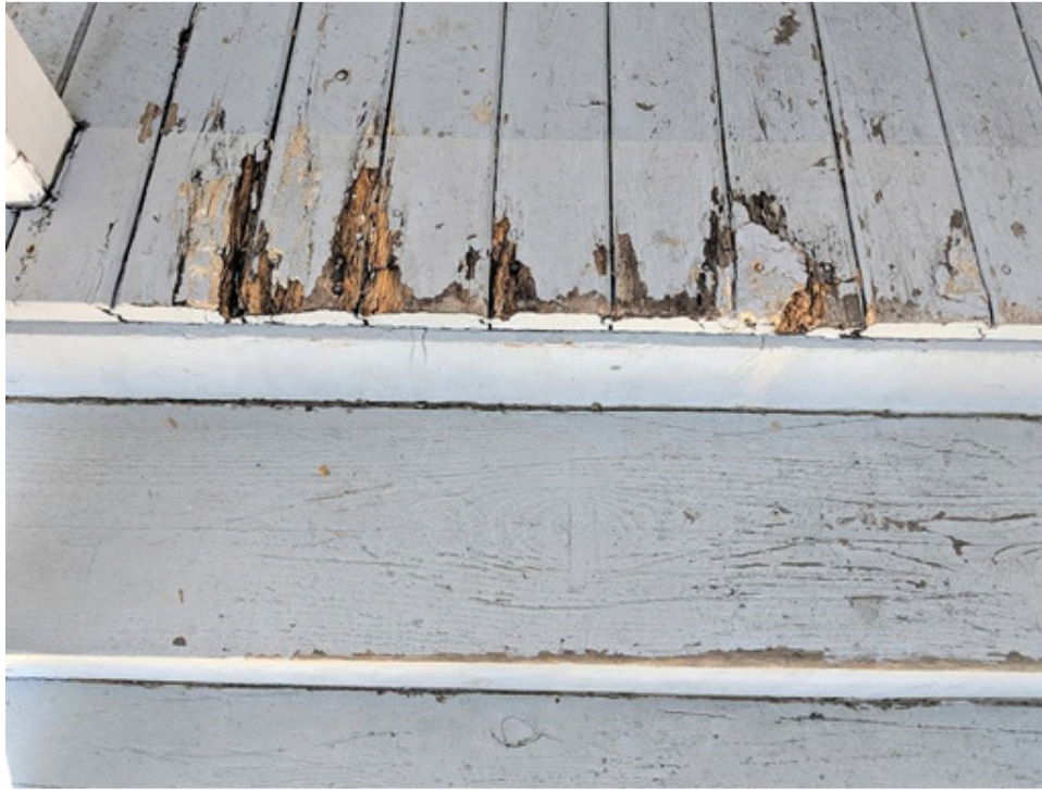
Rotted tongue and groove floor boards located on the front porch.
