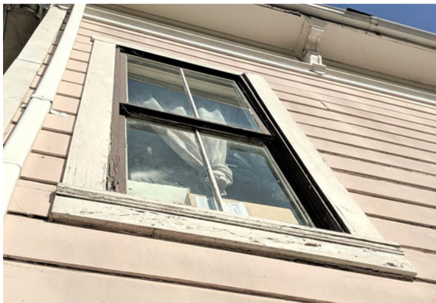
Fogged window and dry rotted window sash.
