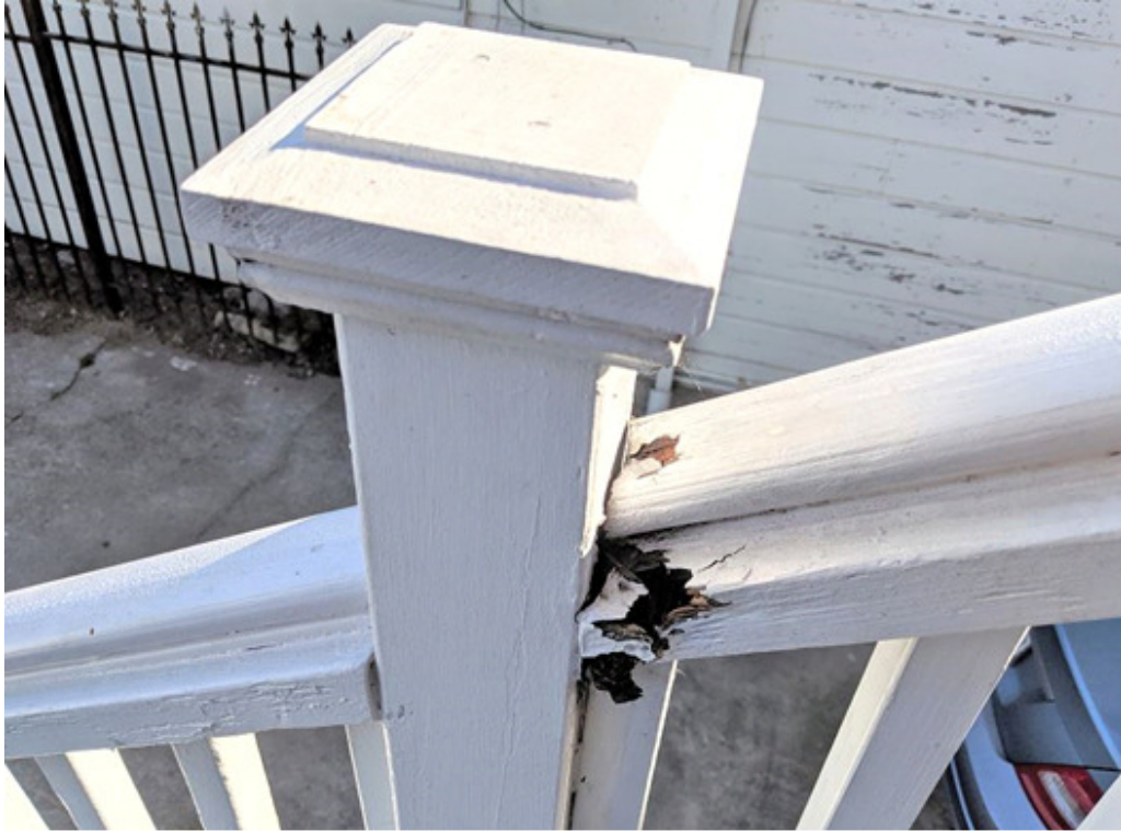
Dry rotted hand rail on the front staircase. Most of the structure is rotted, and so the entire front staircase needs to be rebuilt.
