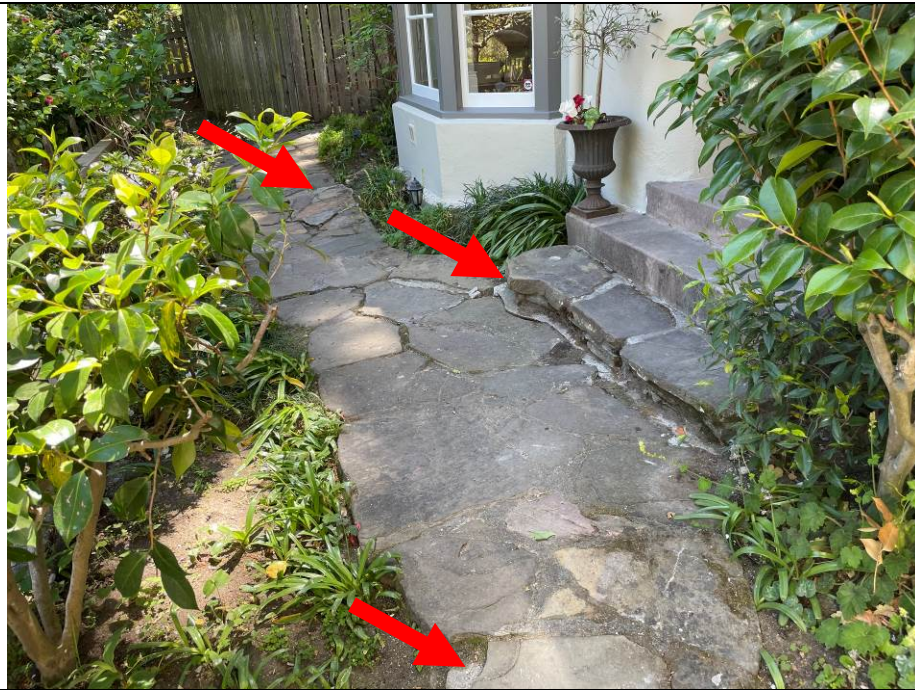
Work Item #4 - Photo 3 Red arrows show missing and or significant separation based on ground settling.
