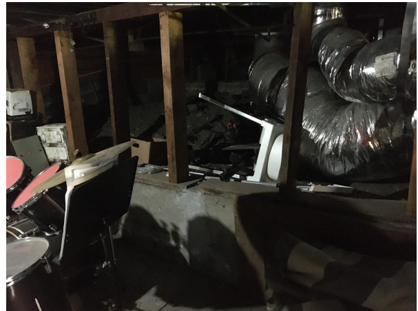
shear panels to be added to cripple walls, current support beams are leaning
