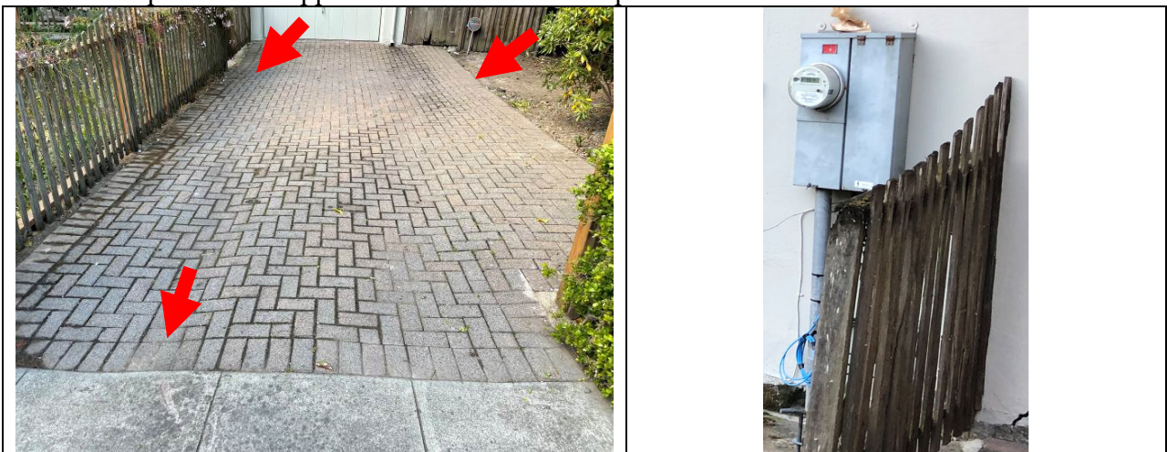
Work Item #9 - Photo 1& 2 1990's era concrete brick driveway to be repaired. High spots and valleys are present. Sewer line underneath to be replaced. (If this was concrete it would be severely cracked but the brick helps conceal the soft sediment deformation. Exposed utility box.
