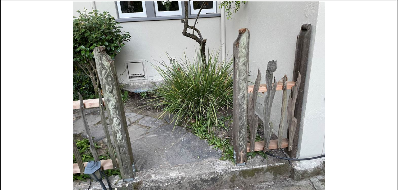
Work Item #2 - Photo 3 Example of rose garden fence and posts carved and mounted to the house. Several fence items are damage or missing.
