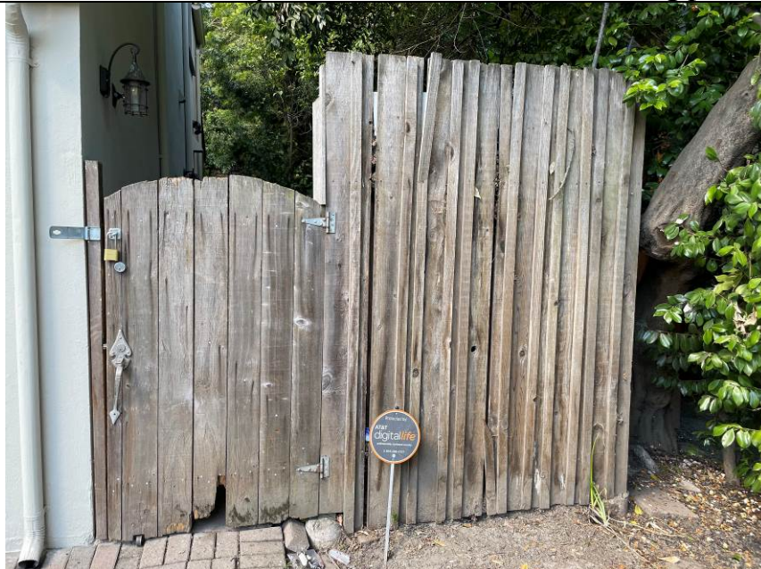
Work Item #3 - Photo 2 Right front garden fence front elevation. Fence has wood rot and missing panels.
