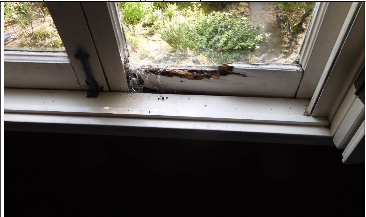
Work Item #2 - Photo 1 Second Floor Window with dry rot and slipping window panes.
