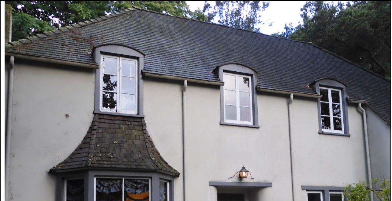
Work Item #4 - Photo 1 Replace wood shingle roof with new fire-retardant rated wood shingle roof on upper & lower portions. Wood roof dated early 1990s.
