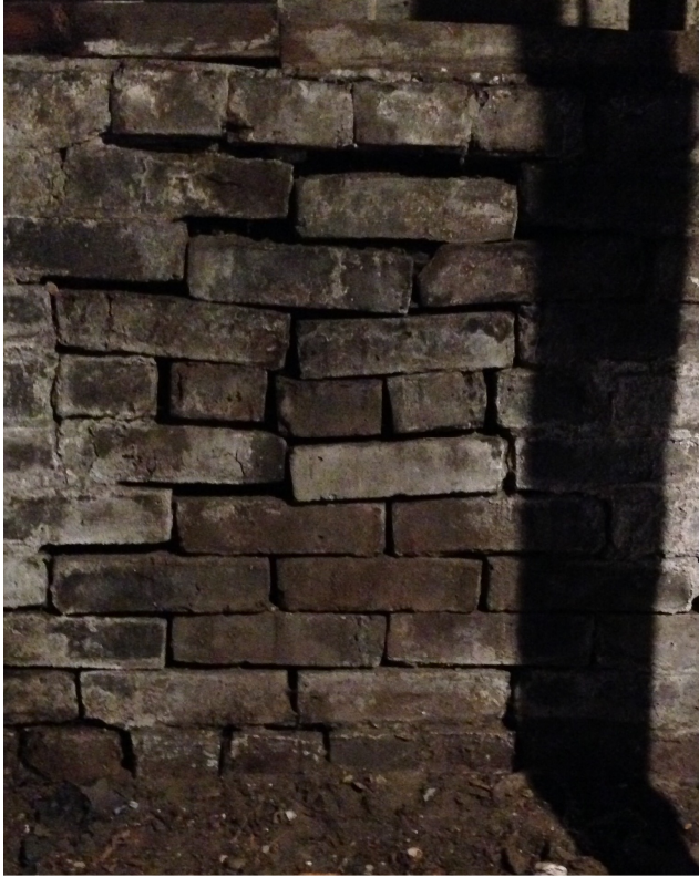
Fissures in the brick foundation
