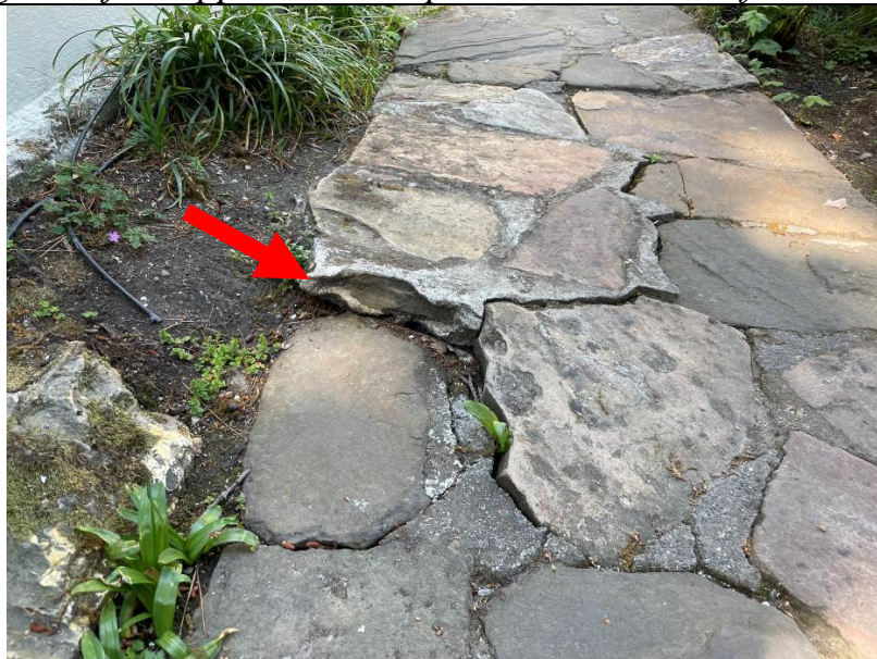
Work Item #4 - Photo 2 Red arrow depicts significant separation based on ground settling.
