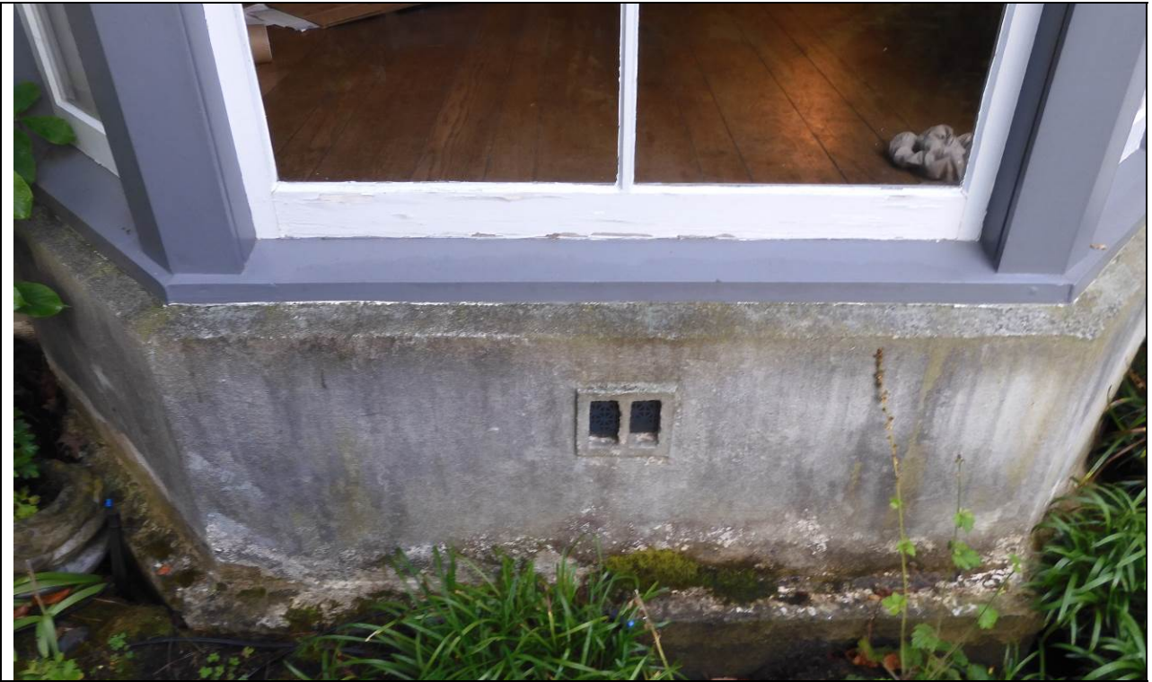
Work Item #2 - Photo 2 Rehab and restore the front elevation oriel style bay window on the first-floor eastern elevation.
