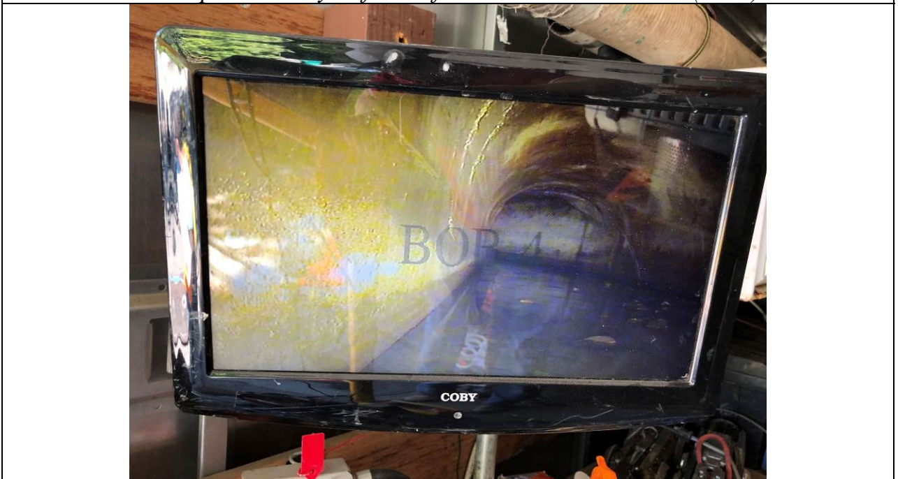
Work Item #1 - Photo 3 Robot "BOB-4" with camera. TV view of the poured concrete 100 plus year-old culvert directly under 901 Trestle Glen Rd (2019). Install three grade beams to further separate the house from the culvert 17-ft below the house grade level.
