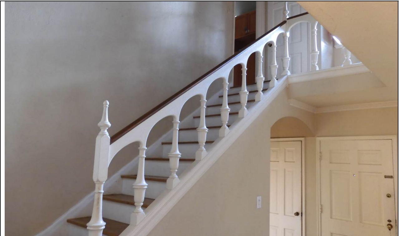
Work Item #1 - Photo 4 Interior original staircase cracking due to settling. Foundation repair to stabilize.
