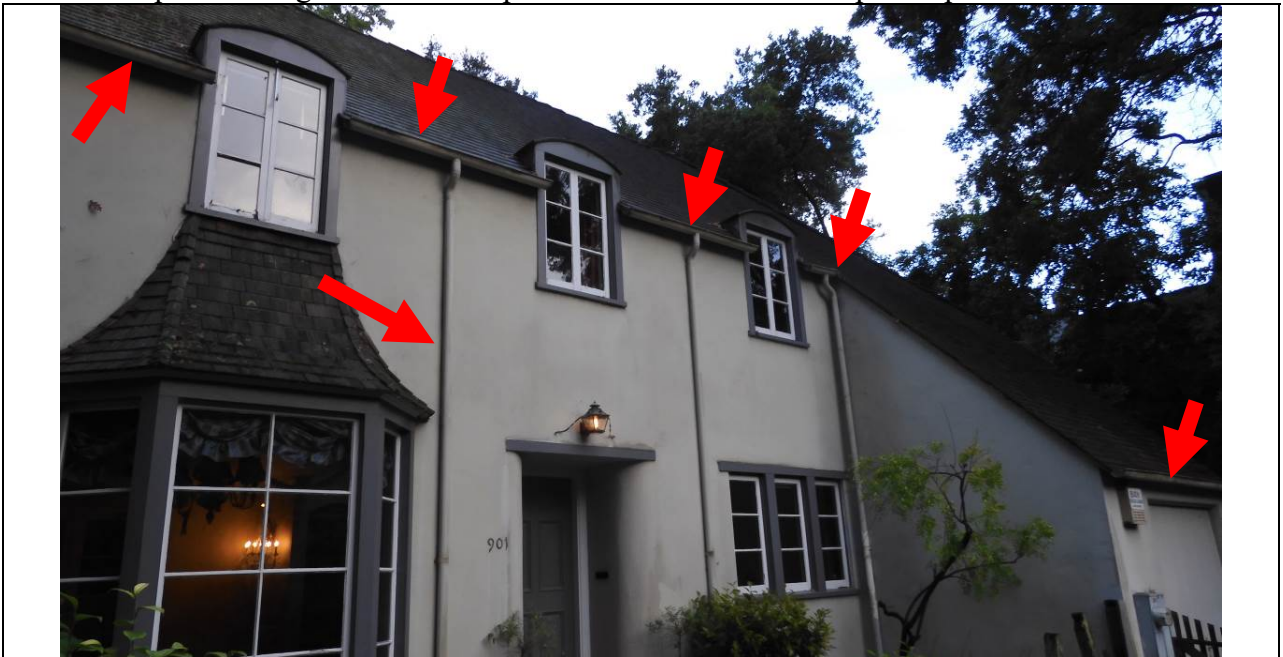
Work Item #7 - Photo 1 Historical gutter and downspouts to be repaired and/or replaced.
