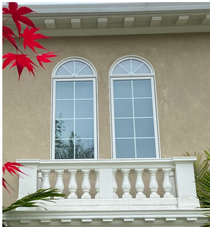
Work Program Item #2 Figure B: Two full-height narrow casement windows with overlying fanlights
