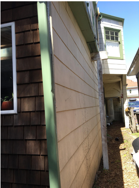
asbestos shingles along left side of home
