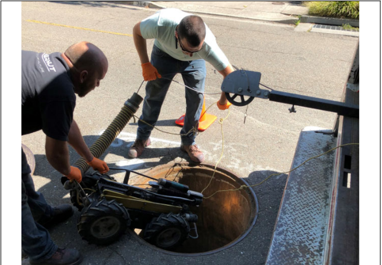
Work Item #1 - Photo 2 Robot with camera entry into Trestle Glen Road culvert access port directly in front of 901 Trestle Glen Road (2019).
