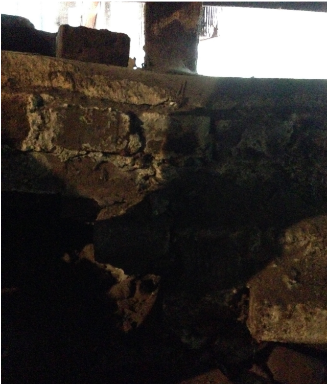
Collapsing sill plate and hollowed out brick foundation
