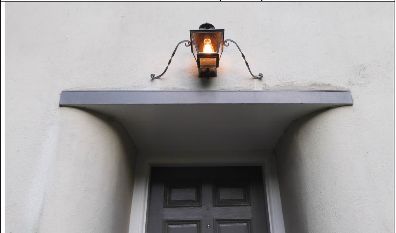
Work Item #2 - Photo 6 Remove repair and rewire original light feature. Exposed wire insulation present. Patch and paint exterior wood and stucco.
