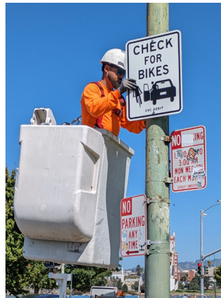
Check For Bikes sign being installed on Lakeshore Ave by the Traffic Maintenance team of OakDOT's Safe Streets Division
