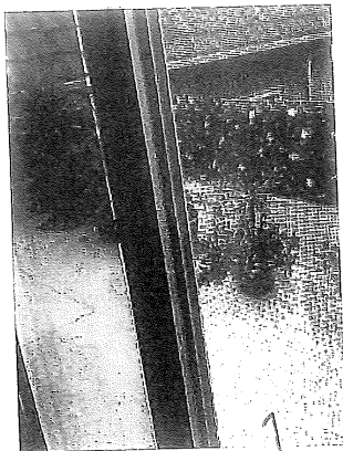
bedroom vent no evidence of leak.
