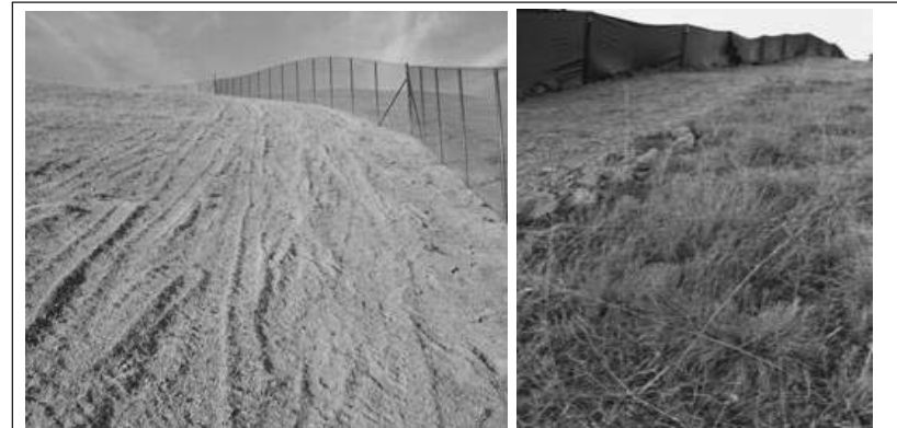
Figure 1. Example of unauthorized damage to former rare native grassland and Alameda striped racer habitat torn up during construction of perimeter fence ( left ) and wildlife exclusion fence ( right ).
