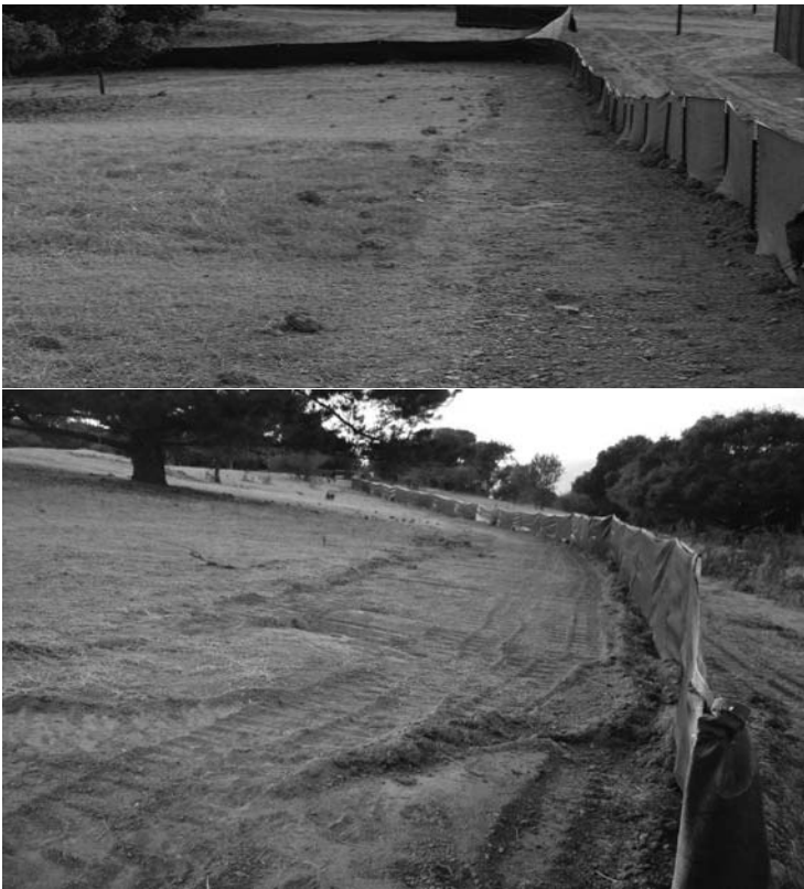
Figure 6. (top) EBZS trenching and scraping damage across original and intact native bunchgrass prairie for the wildlife exclusion fence. (Site Areas D–E). Approximately 1,700 linear feet x 7 feet = estimated .27 acres damage outside of project footprint. Complaint sections 1a–c, g, h; 2b, c, d. (bottom) Another example of the damaging method used to install the wildlife exclusion fence.
