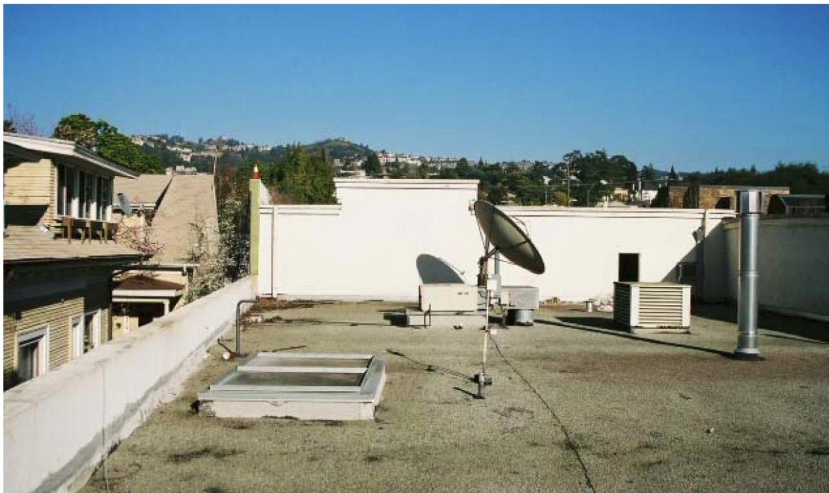
4 Mechanical Equipment and Ventilation Louvers on Existing Store Roof
