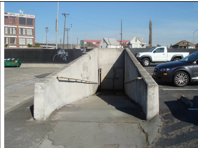
Closed I-880 pedestrian undercrossing at Livingston Street
