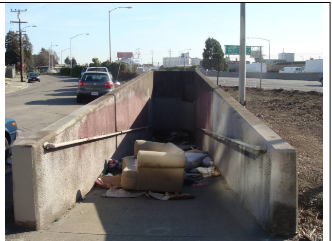
Closed I-880 pedestrian undercrossing at Calcot Place
