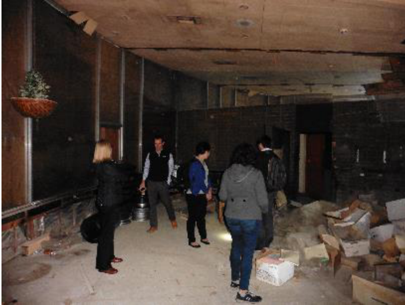
Figure 10: Interior View looking toward former counter at open kitchen (similar vantage point to Figure 7), Page & Turnbull, 2015
