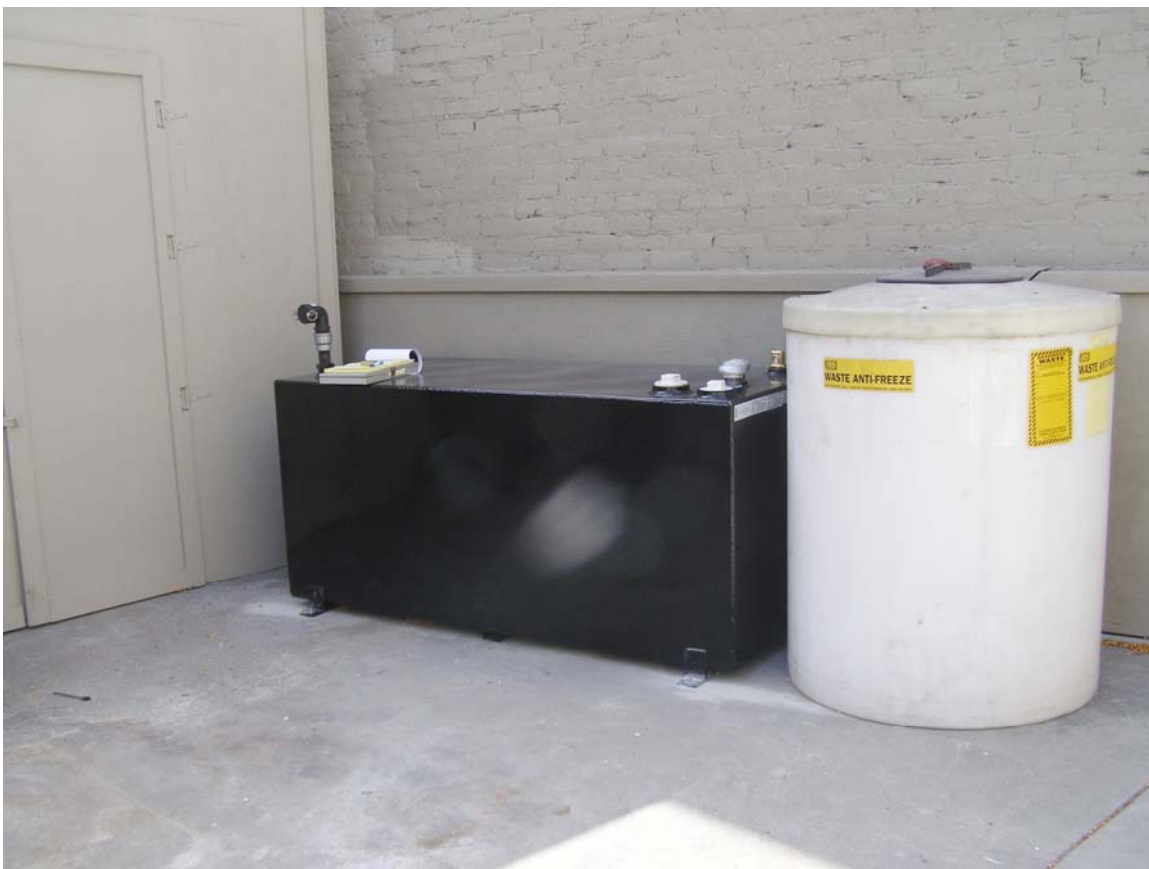
Photograph 5 - View of the USTs for oil and coolant (currently empty and unused)
