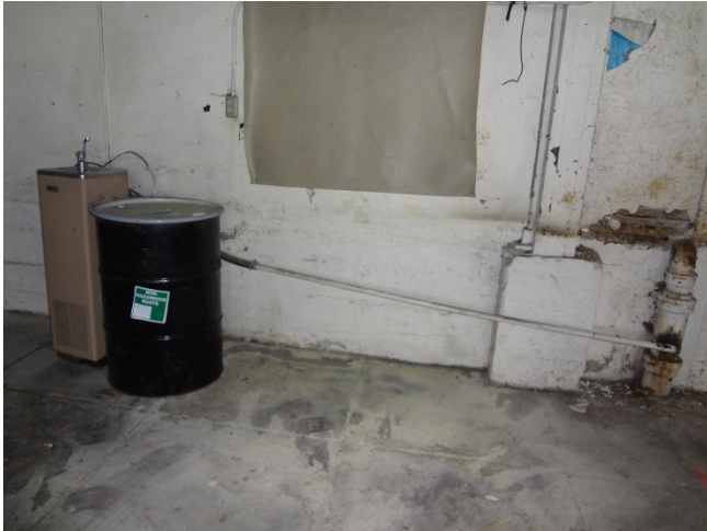
Photo 15: View of unidentified non-hazardous waste drum at 2800 Broadway.
