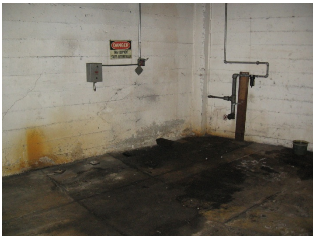
Photograph 5: Significant ground staining was observed in a wash-out area at the northeastern corner of the building.
