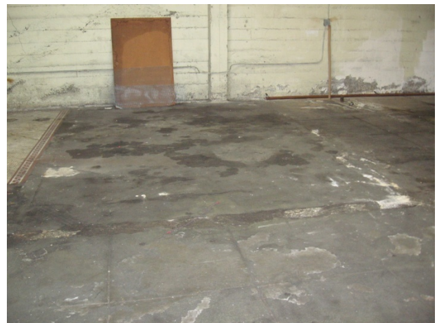
Photograph 6: The northern warehouse portion of the building, adjacent to the showroom floor. An area of patching in the concrete may suggest a potential UST site.
