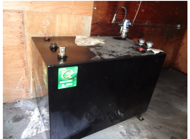
Photo 10: View of fuel AST in shed at 2820 Broadway.
