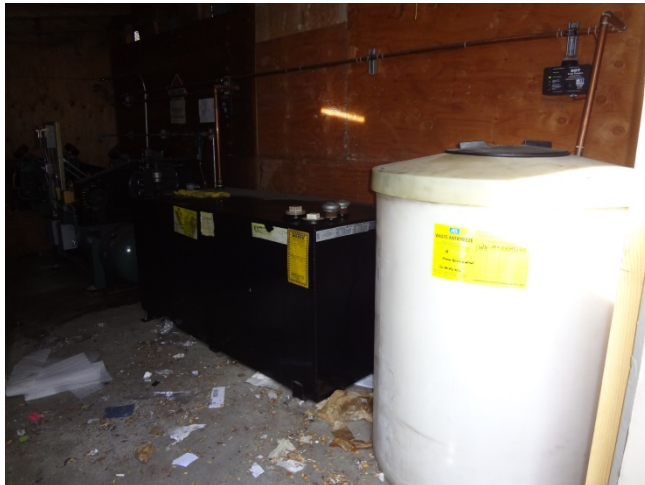
Photo 9: View of waste antifreeze and waste oil ASTs in shed at 2820 Broadway.
