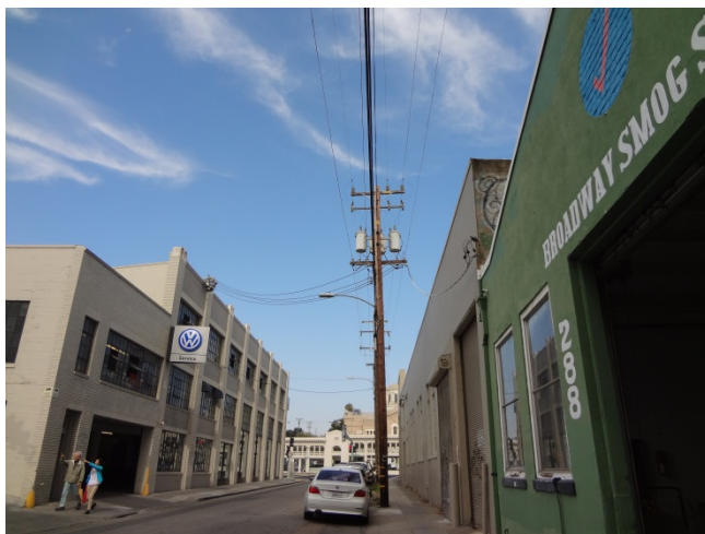
Photo 11: View of pole-mounted transformer on southwestern portion of 2800 Broadway.
