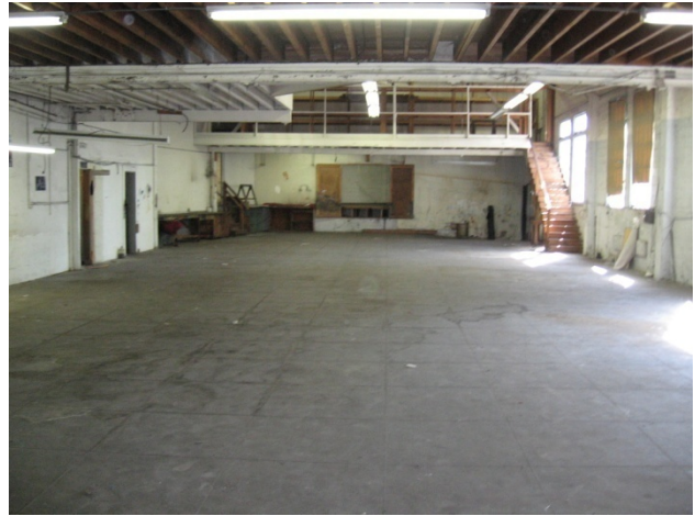
Photograph 8: The southern warehouse portion of the building. The loading dock can be accessed through an opening in the east wall.
