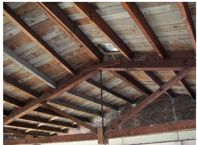
Photograph 12: The roof structure above the showroom has redwood-framed trusses. The gable end consists of bricks. No insulation was present.
