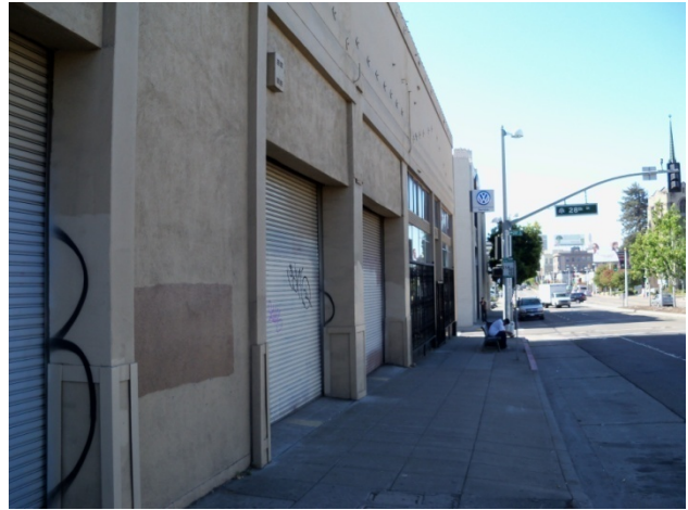
Photograph 2: The rollup doors and showroom windows along the Broadway side of the building.
