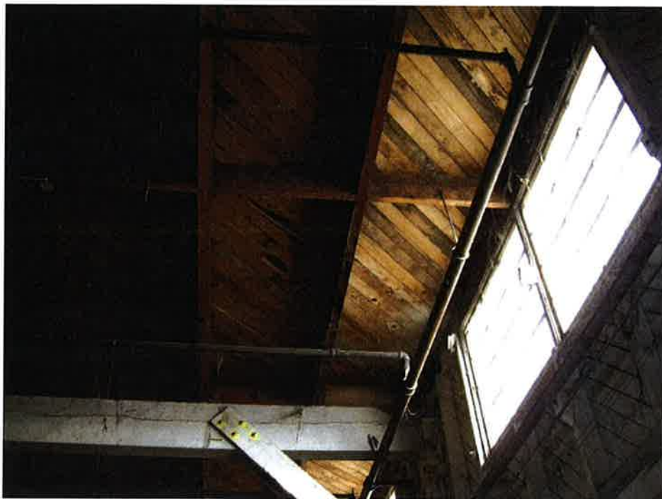
Photo 12: Leak at Roof
