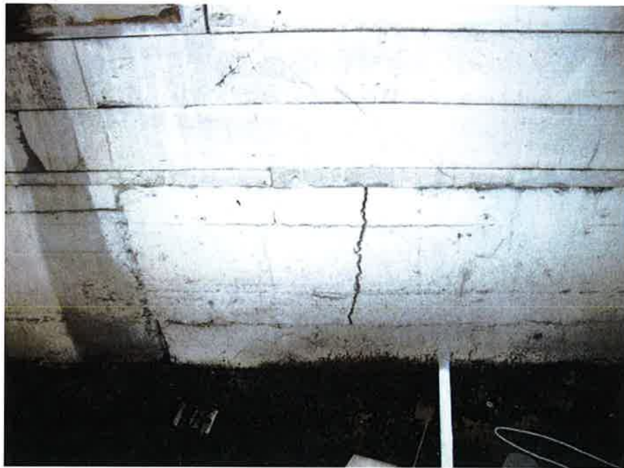
Photo 9: Cracking at Stem Wall (Interior)
