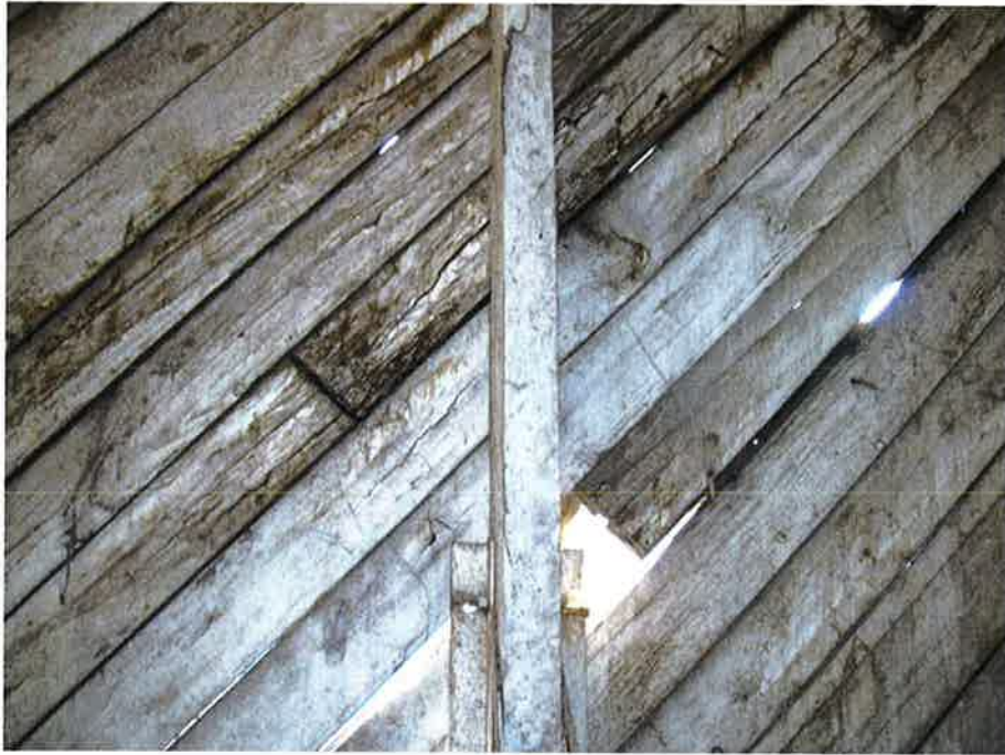
Photo 11: Water Damaged Sheathing
