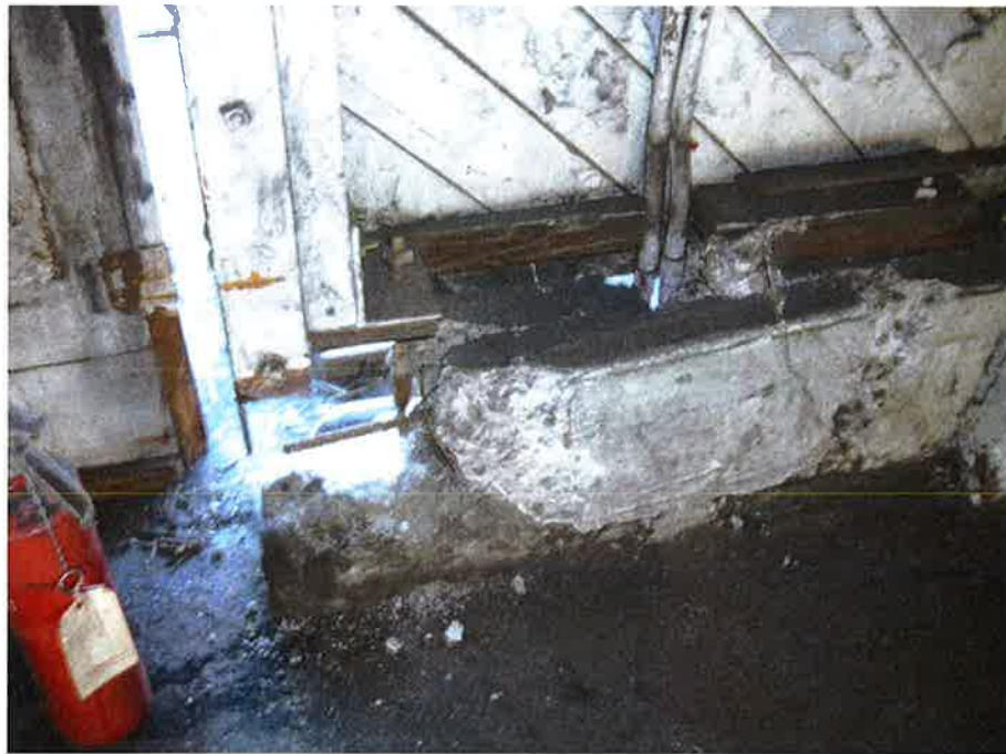
Photo 7: Damaged Stem Wall at Door
