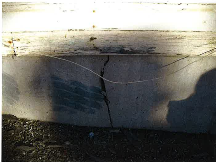
Photo 10: Cracking at Stem Wall (Exterior)
