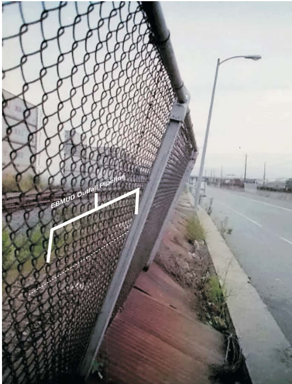
Geologic and seismic damage along the northern boundary of Burma Road in the Gateway development area. To the left is a fence and sidewalk, demonstrating that substantial settlement has occurred in the area. The top of the East Bay Municipal Utility District outfall pipeline is to the left of the fence. This pile-supported structure has remained stable, while surrounding fill has not.
