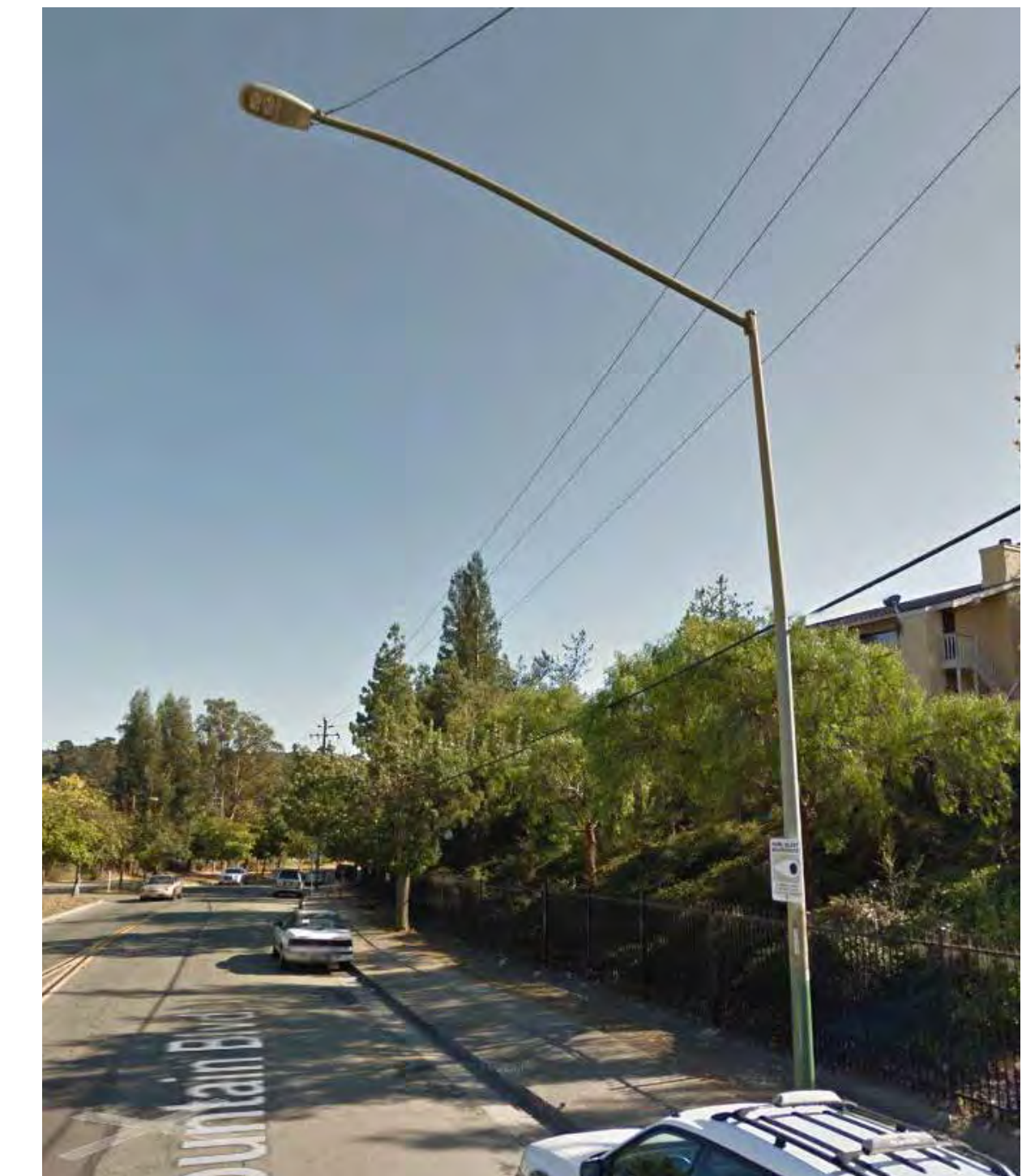
Existing Cobra Head Street Lighting to remain on west side; east side entries only
