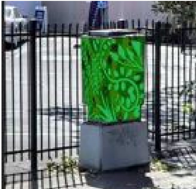
Untitled utility cabinet mural design by BAMP proposed for 8 th St and Adeline St
