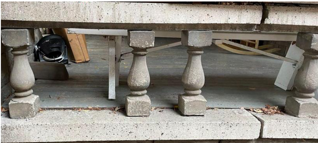
Detail of balustrades and masonry on East (left) and North (right, bottom) sides of porch New balustrades will need to be formed and poured, potentially taller to meet code
