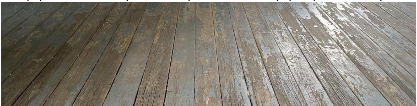
Front Porch deterioration due to unprotected weather exposure (facing Ayala)
