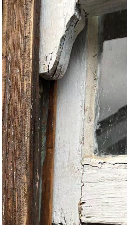
Deteriorating window sash frame and casing at S. side
