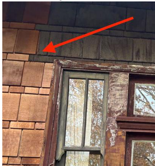
Siding to be replaced (facing Ayala Ave)
