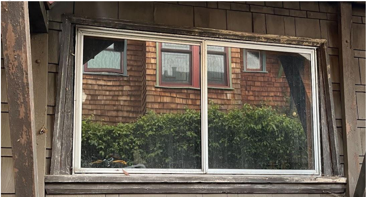
Replace 1 downstairs (North side) large aluminum window with main window and smaller windows on each side
