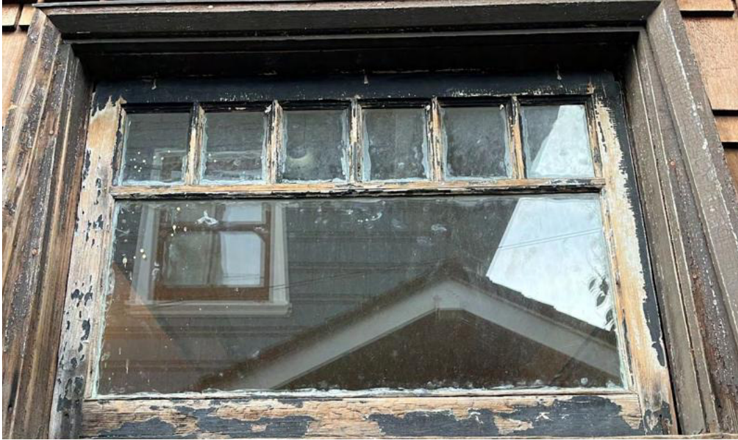
Deteriorating frame of awning window (S. side)
