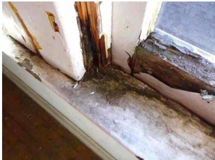
Water damaged interior frame and casing at E. side
