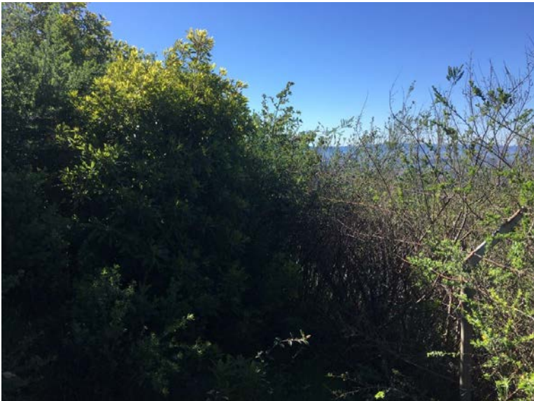
3. Overgrown landscaping downslope from pool patio, with perimeter chain-link fence. .
