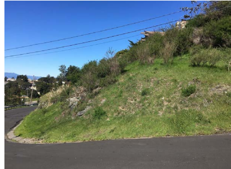
4. Non-native grassland and French broom above serpentine cut slope on shoulder of Old Redwood Road.
