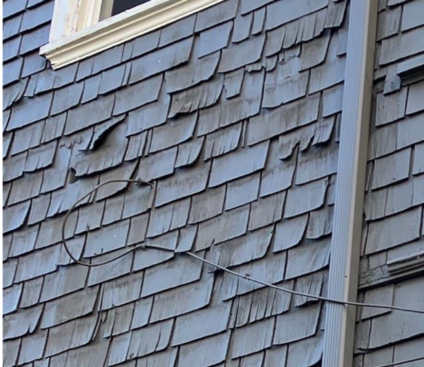
Photo #10 - Shingles from Northeast section of house
