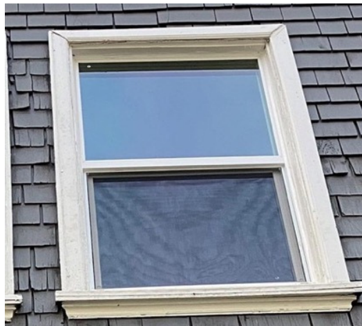
Photo #1 - Original Window Trim (with vinyl sash)
