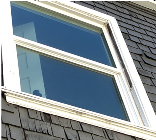
Photo #2A - Original Window Trim (with vinyl sash)
