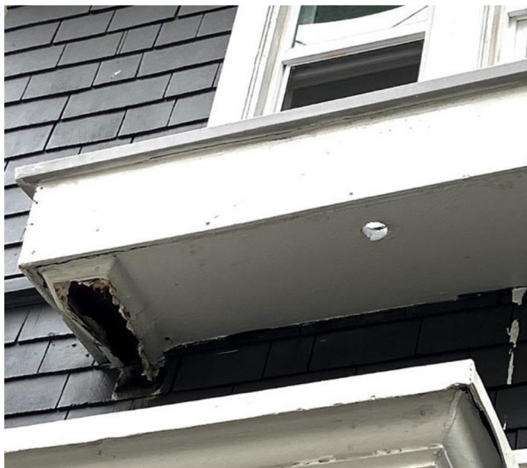
Photo #6 - Missing flower box corbel
