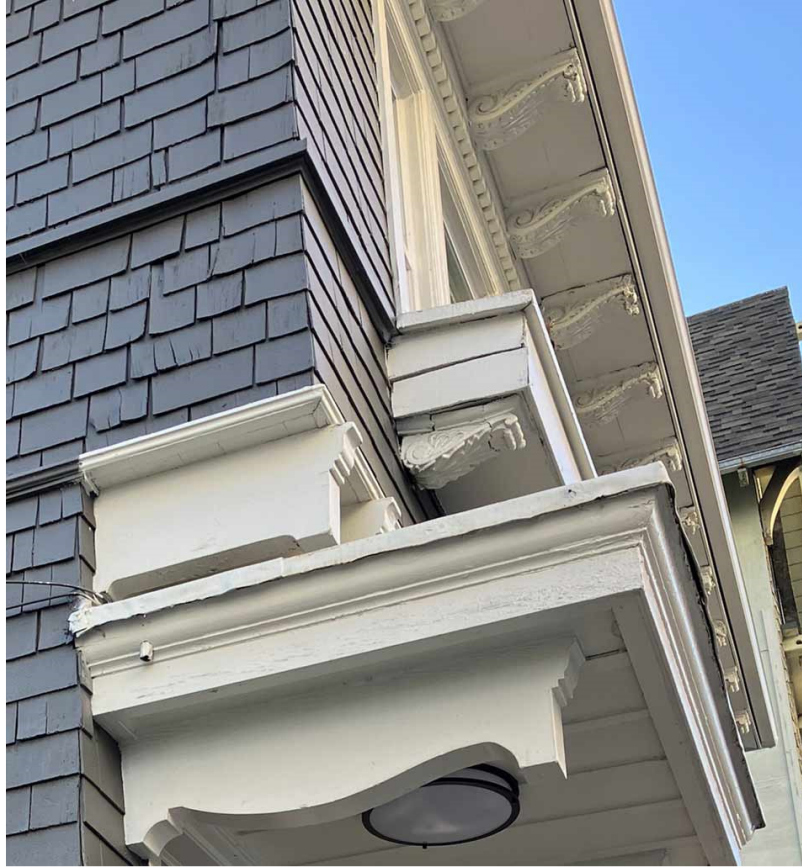
From top to bottom: Eave corbels, dentils, flower box, flower box corbel, cantilever brackets, door overhang
