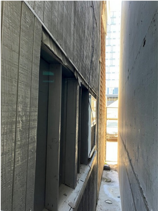
Rear (south side) of house with newly constructed rear staircase walls clad in shingles
