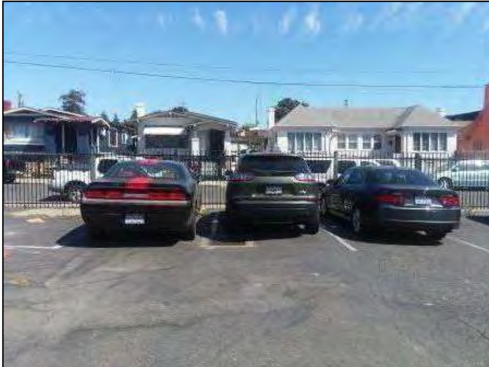
16 : 1409,1415 Mitchell Street - Storm drain in parking lot, photo oriented towards the southeast.
