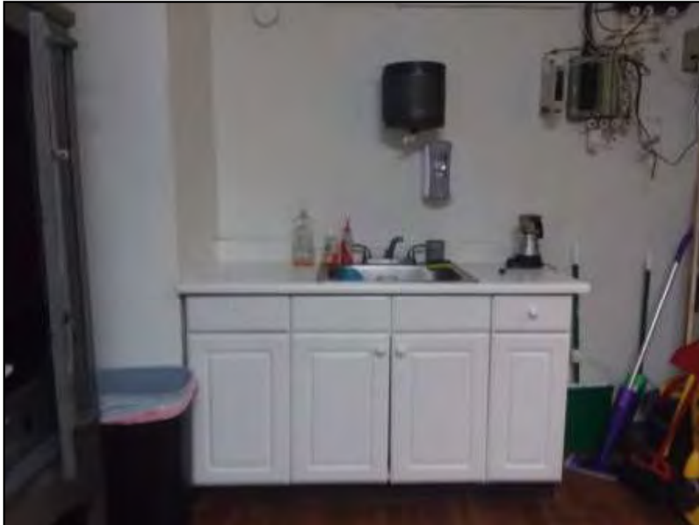
10 : 2716 International Boulevard - Janitor/Server room.
