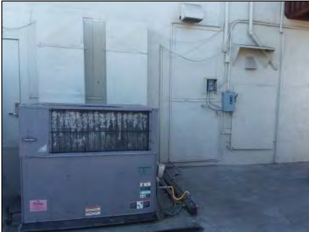
9 : 2716 International Boulevard - HVAC system on northeast exterior of building.
