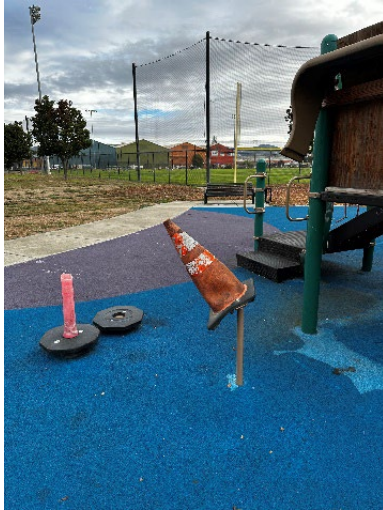
Cones bolted over playground equipment presumably to cover hazardous edges
