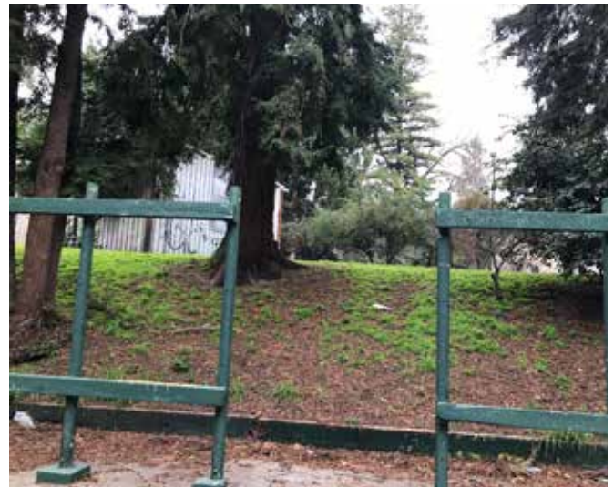
EXISTING FRAME IS IMPORTANT INFRASTRUCTURE
