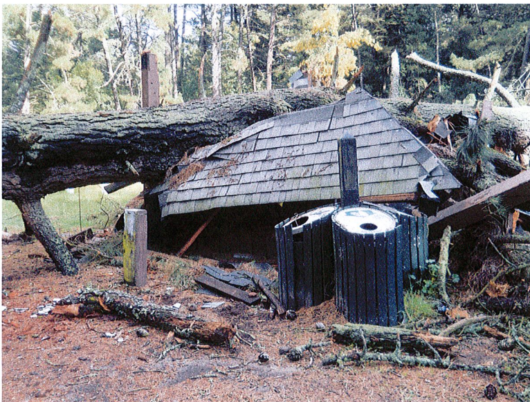
Figure 11: Original announcer's booth squashed by a falling Monterey Pine in 2012. Non-native trees frequently fall in and around Joaquin Miller Park.
