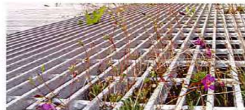
METAL GRATE LID AT BIORETENTION BASIN
