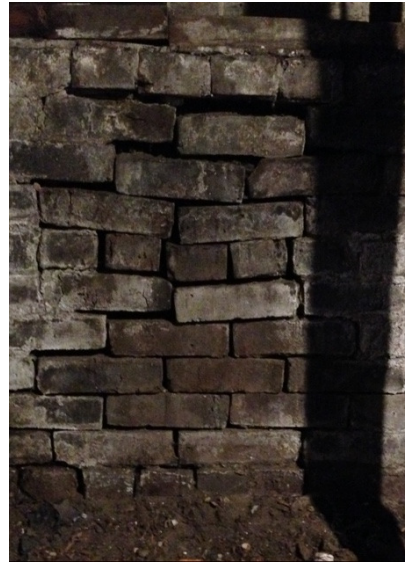
Fissure on brick foundation
