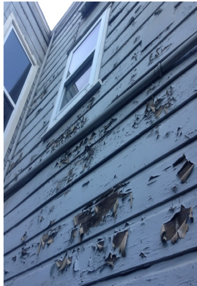
Peeling paint on south side of house
