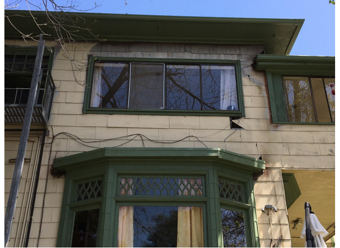
original bay window in bottom story compared to vinyl windows in the top story (right/SW side)
